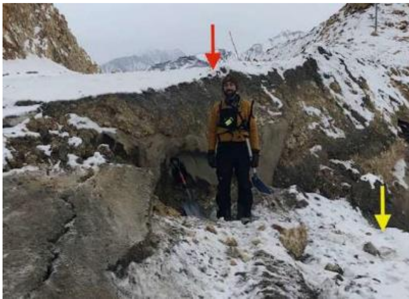
Figure 4. Pretty Rocks Landslide scarp at the Denali Park Road in November 2019 (National Park Service 2020). The road had been displaced approximately 10 ft. since September 2019 (from red arrow to yellow arrow).
