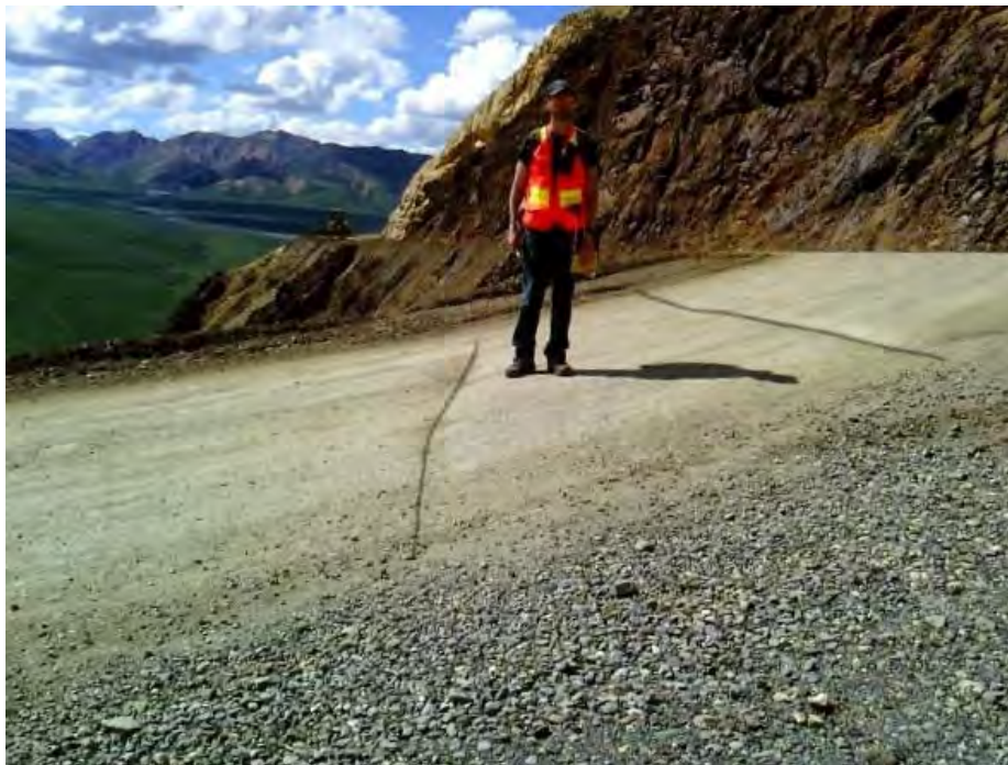
Figure 18: Western road cracks. The crack on the right is longer, more prominent, and was visible more often during field work. Highlights added for clarity, but do not represent extent of cracks. Photo taken looking southwest.
