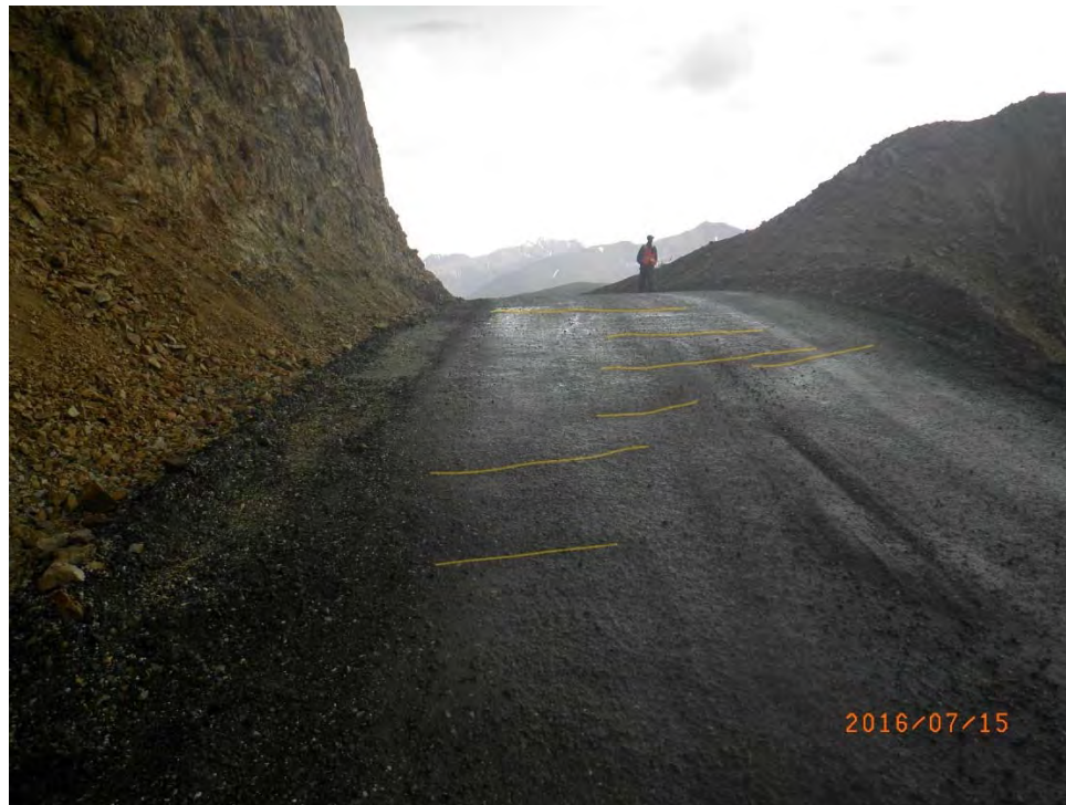
Figure 20: Eastern, en echelon road cracks. Highlights added for clarity. Photo taken looking east.
