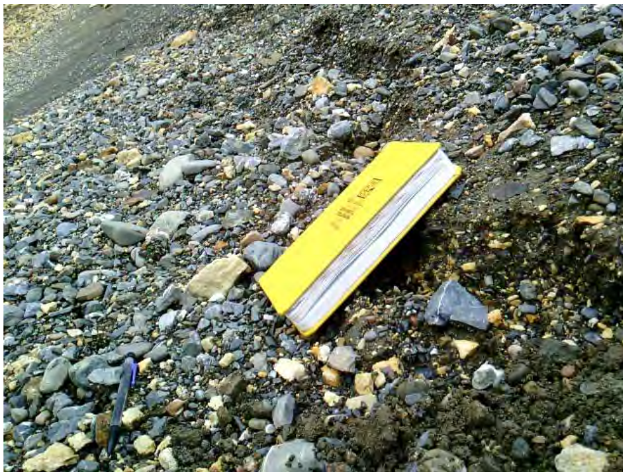
Figure 22: Crack directly below the road which developed during field work (July 2016). Coincides with band of significantly increased elevation (Fig. 5). Photo taken looking west.
