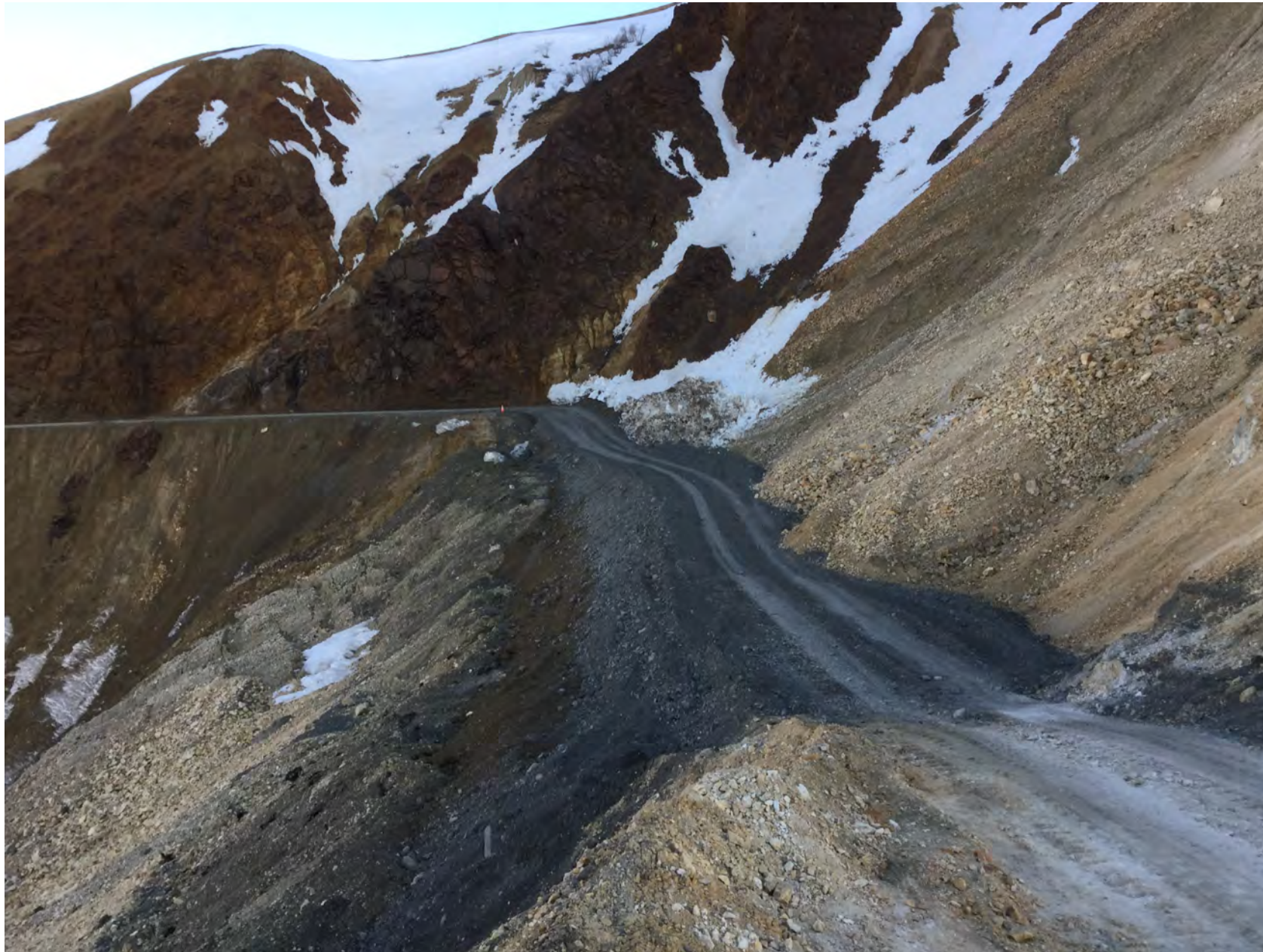
Figure 11. Site photo at the rebuilding of the road grade as it is brought to grade on April 29, 2020.
