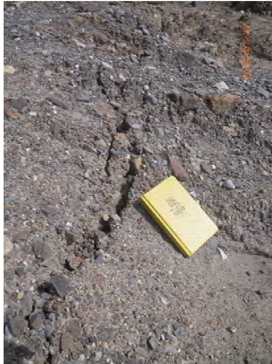
Figure 19: Detail of western road crack. Offset varied based on road maintenance and precipitation.
