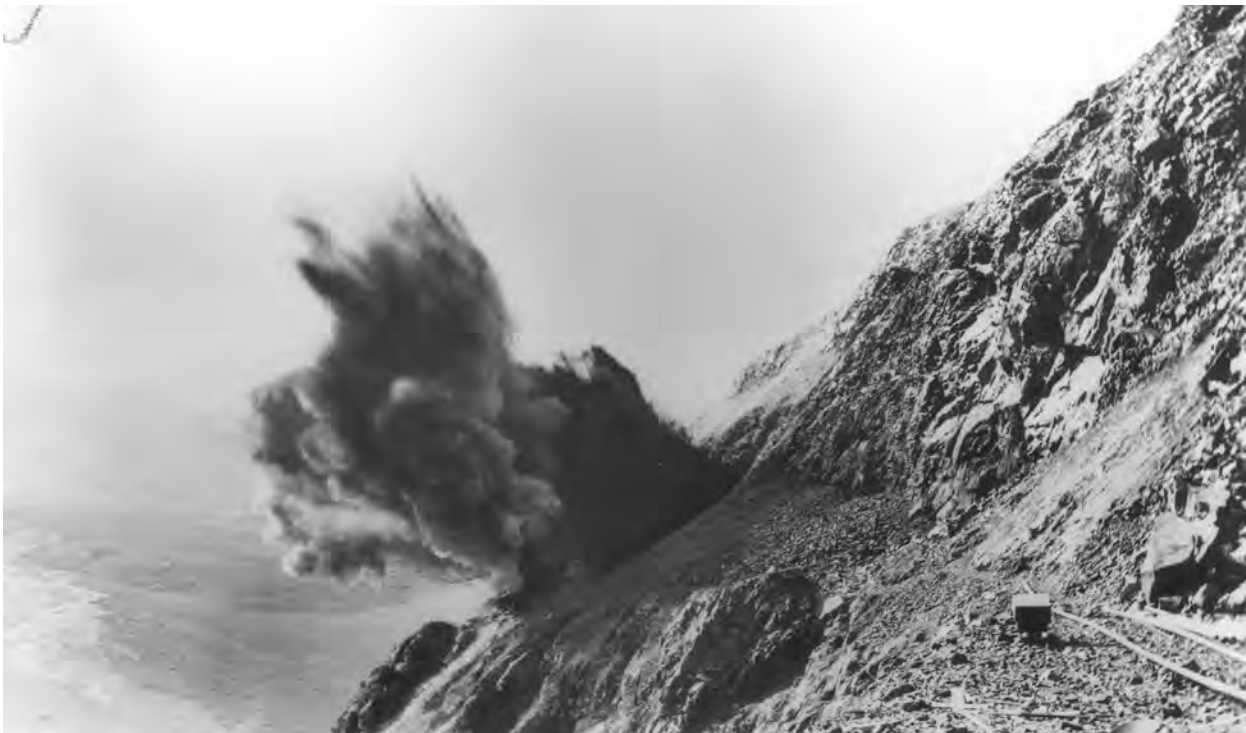
Blasting the High Line route (Alaska State Library, Alaska Road Commission Collection, 61-18-127).
