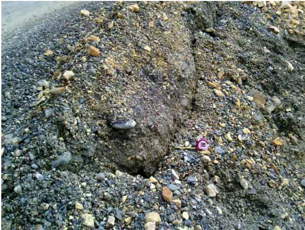
Figure 21: Detail of eastern road crack where it continues below the road and turns easterly to propagate parallel to the road surface. Offset averaged 1 ft. Photo taken looking east. Tape measurer for scale.
