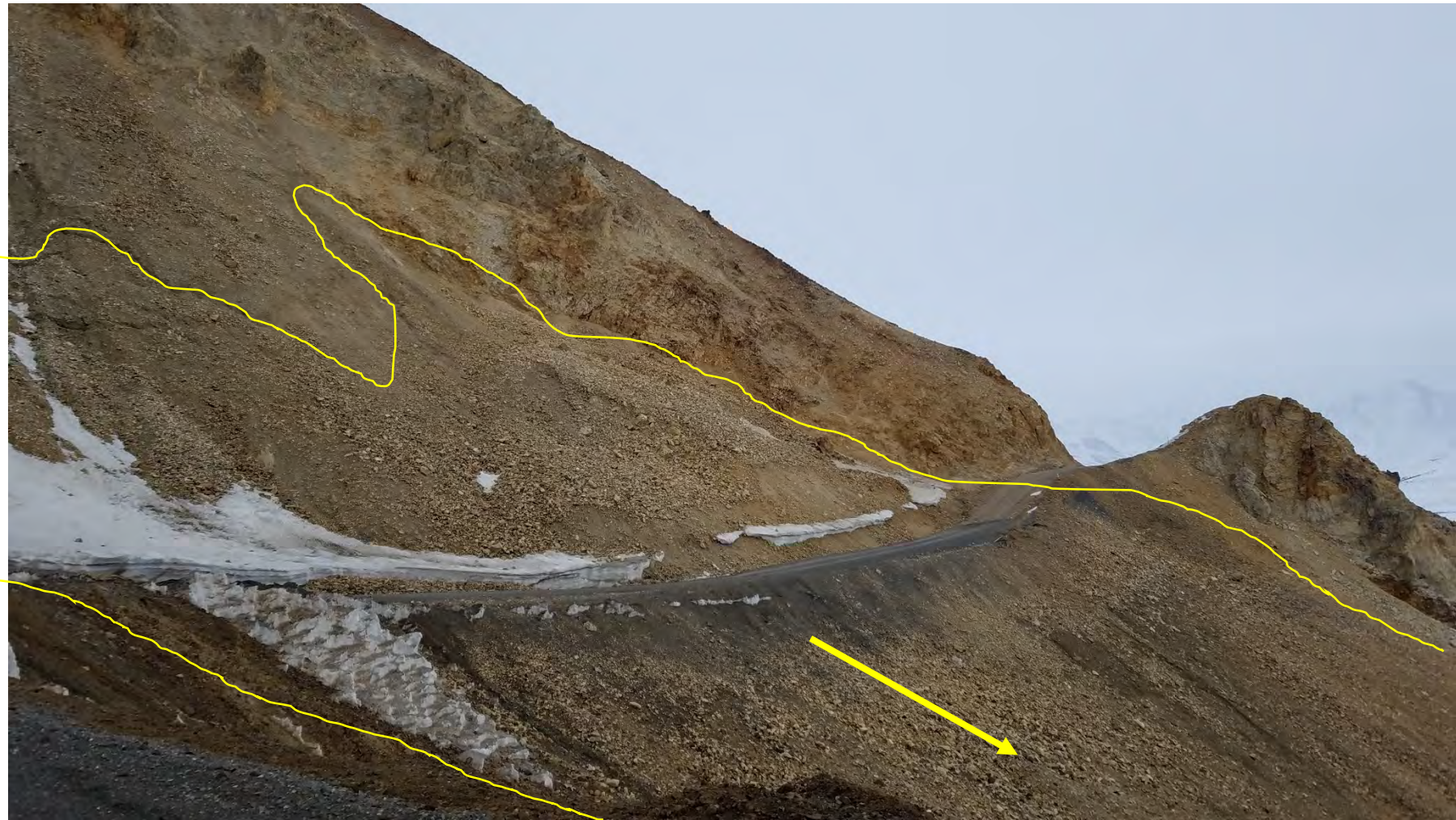
Figure 5. May 2018 Landslide headscarp and lateral scarp limits at road before Maintenance day labor project.
