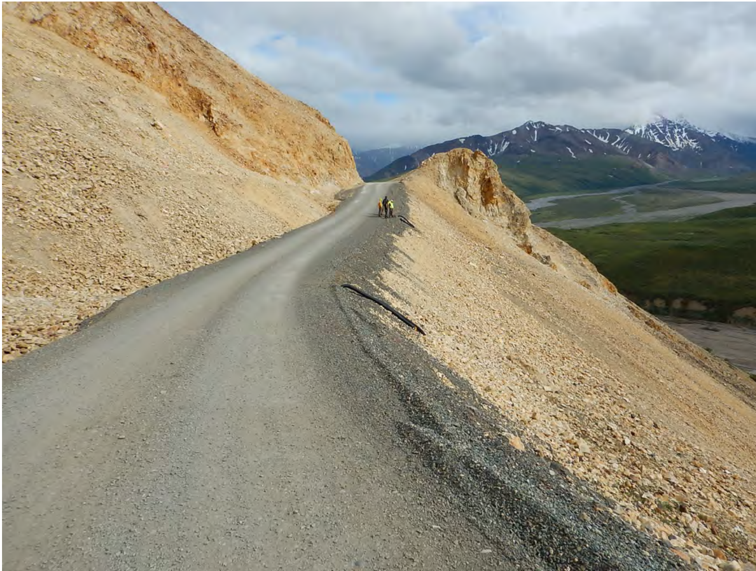
Figure 6. May 2018: After deep patch construction and conduit installation for drilling and instrumentation program
