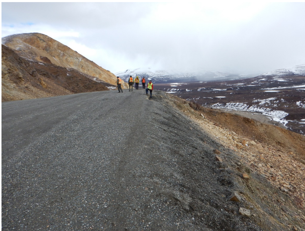
Figure 5-19. Looking east at slump during road opening in May 2019. FHWA photo, 2019.
