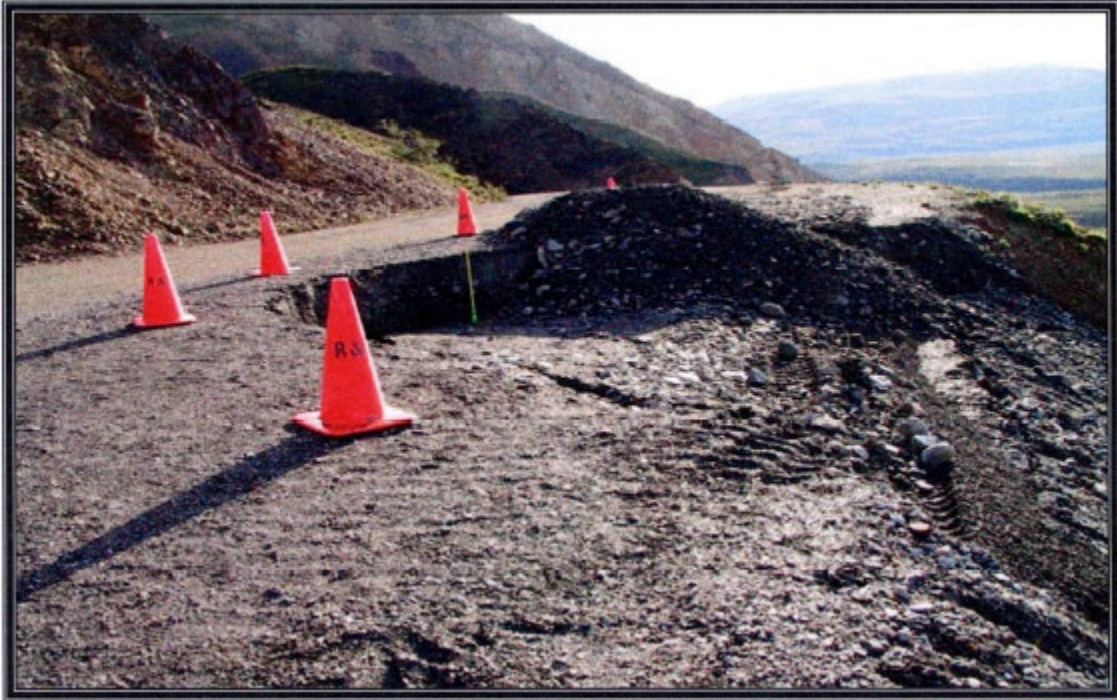
Figure 5-17. Looking east at slump on August 18, 2003. NPS/Martin Grosnick photo.
