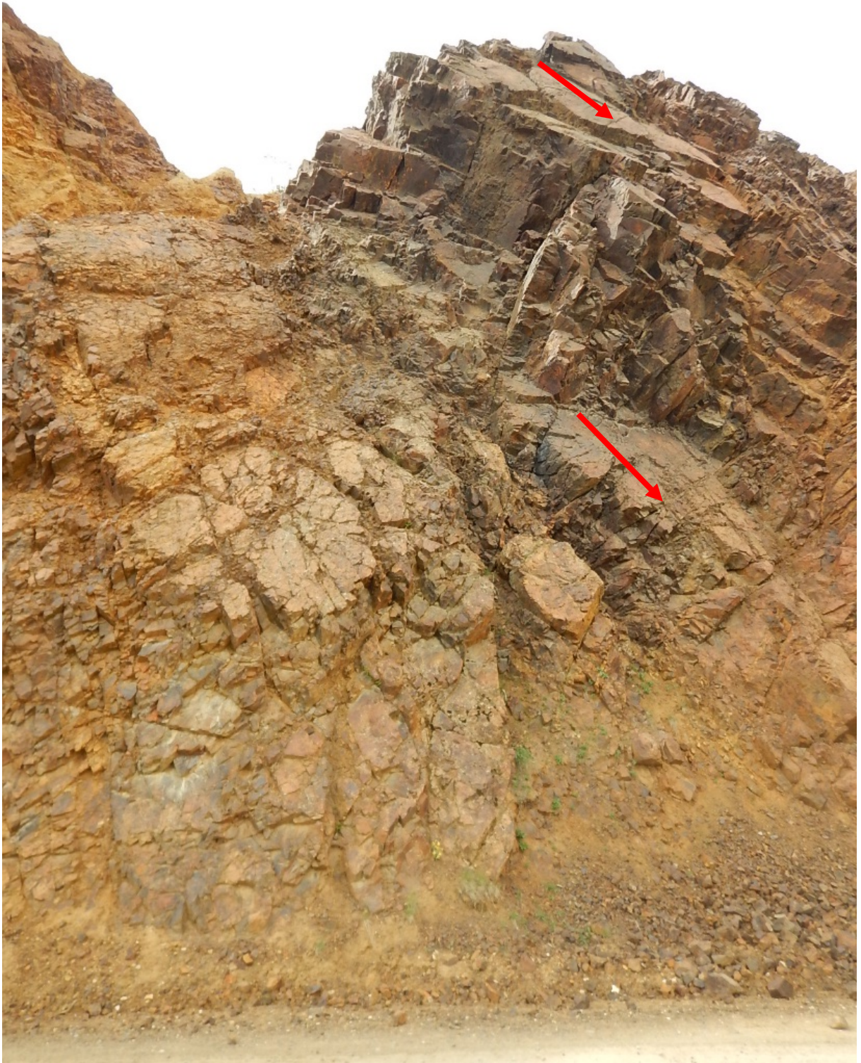
Figure 5. Photograph of the basalt bedrock outcrop at the approximate location of the west bridge abutment. Red arrows show the direction of the controlling discontinuity.
