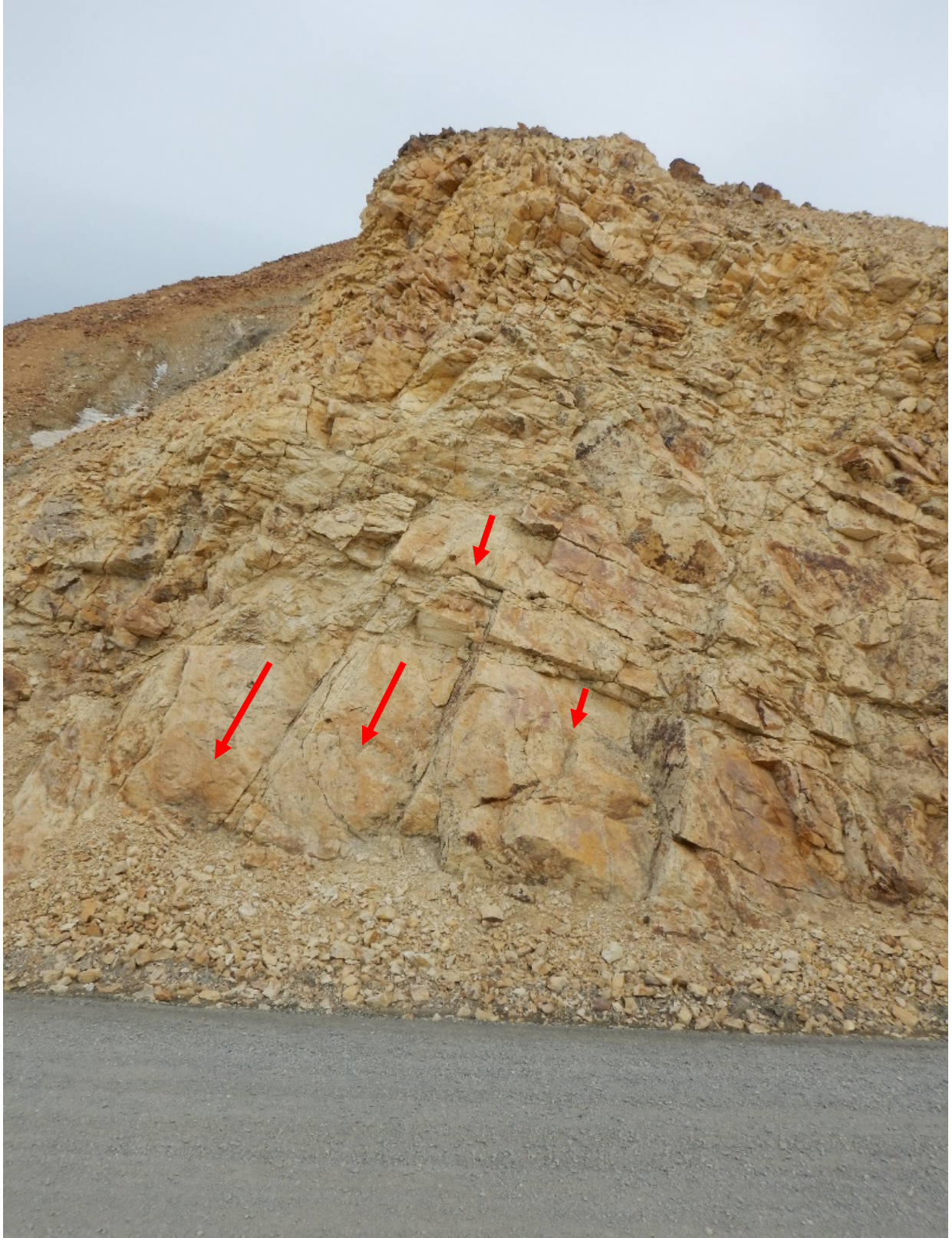
Figure 3. Photograph of the rhyolite bedrock outcrop near the east bridge abutment location. Red arrows show the direction of the controlling discontinuity.
