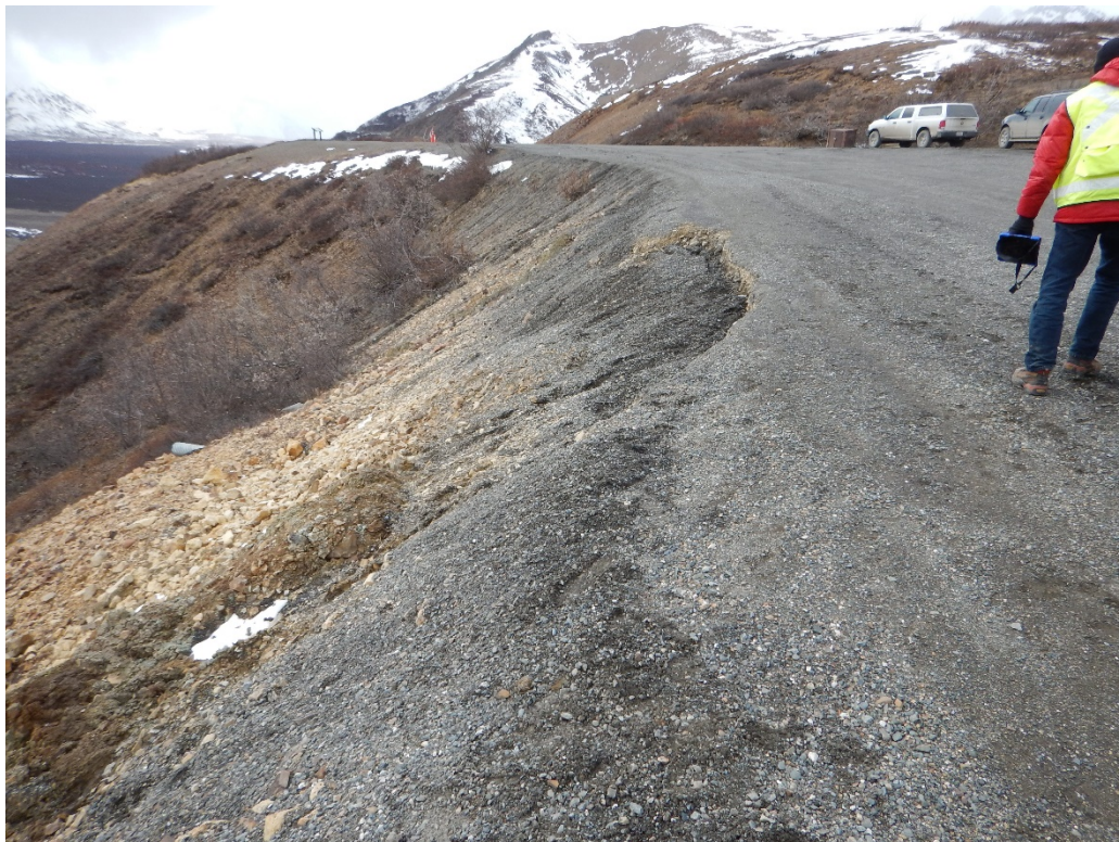
Figure 5-18. Looking west at slump during road opening in May 2019. FHWA photo, 2019.
