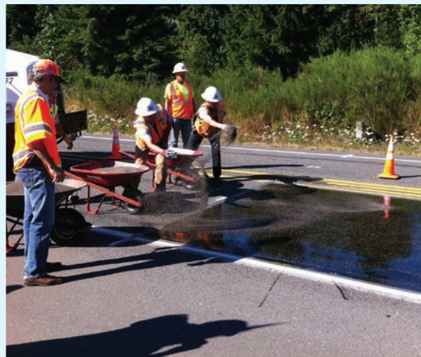
Installation of high-friction surface treatment (HFST) – example improvement resulting from the county safety program
