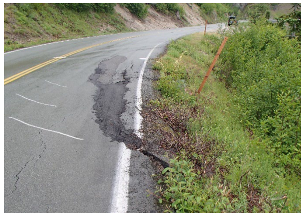
Figure 7: Roadway deformation caused by embankment failure. Forest Service Road 90, Milepost 11.5.
