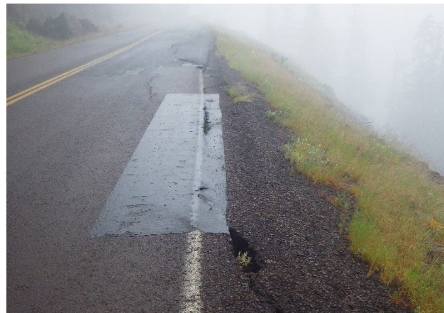
Figure 16. Instability requiring repeated maintenance attention. Forest Service Road 25, Milepost 25.
