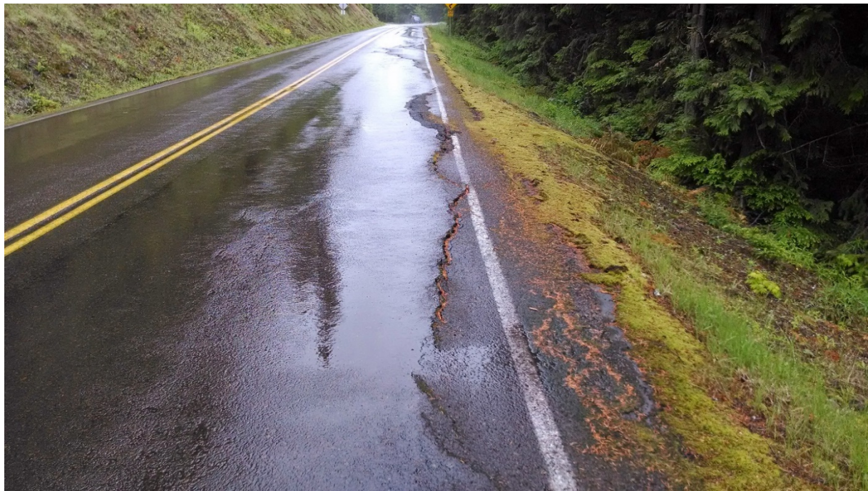
Figure 5. Embankment failure affecting up to 25 percent of the roadway. Forest Service Road 25, Milepost 30.
