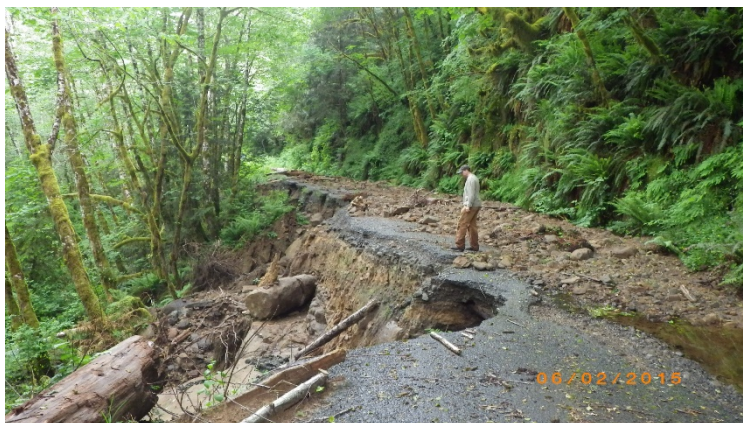
Source: BLM Figure 7. Landslide on a BLM road, southwest Oregon.
