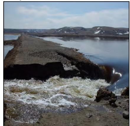
Road damage due to flooding at Arrowwood NWR (top); washed out bridge at Flint Hills NWR (bottom).
