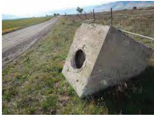
Figure 8. Hazardous roadside object identified through a systemic safety study.
