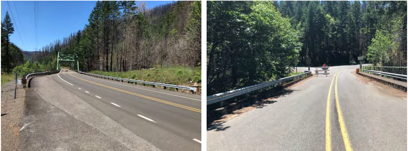
Figure 6: Apparently Undamaged Guardrail and Bridge Rail (OR 224, MP 31.2 and MP 49.97)
