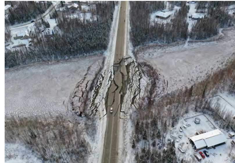
Vine Road 2018 Earthquake Damage. Alaska DOT&PF photo.
