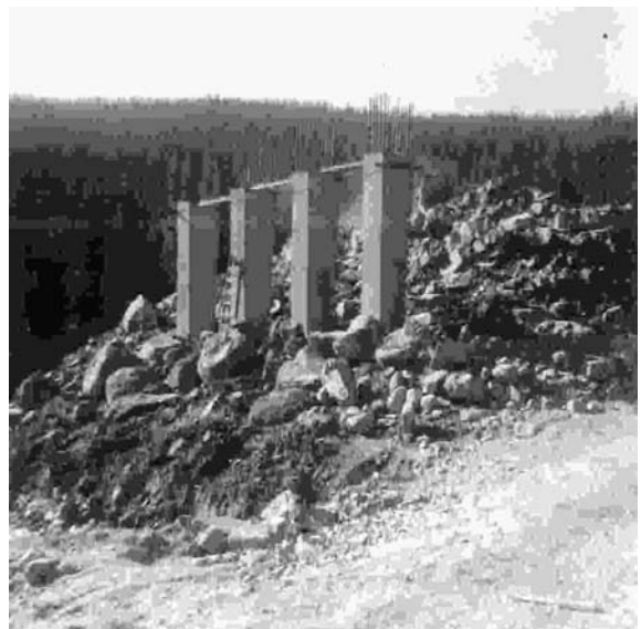
Construction begins for a bridge across the St. Vrain River in Peaceful Valley, Colorado. Photo Courtesy Larry Brown.
