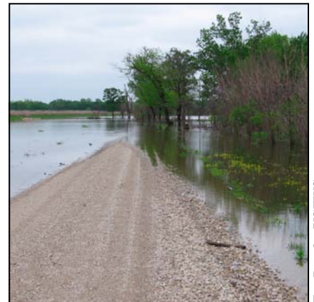
Roads both affect and are affected by hydrology. Floodwaters wash out a road at Flint Hills NWR (top); levee road at Blackwater NWR (bottom).
