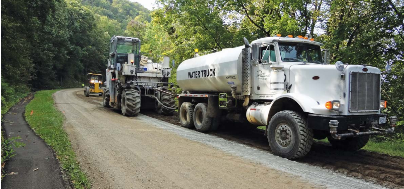
A 4,000-gal Kenworth water tanker makes its way down the Parkway trailed behind by a reclaimer.
