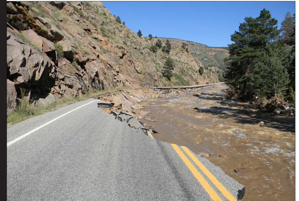
Catastrophic flooding in Colorado's Front Range in 2013 affected many state and county roads accessing national parks and forests. Federal Lands deployed assessment and survey teams to assist the National Guard and Colorado DOT, and also provided engineering and technical support for repairs.
