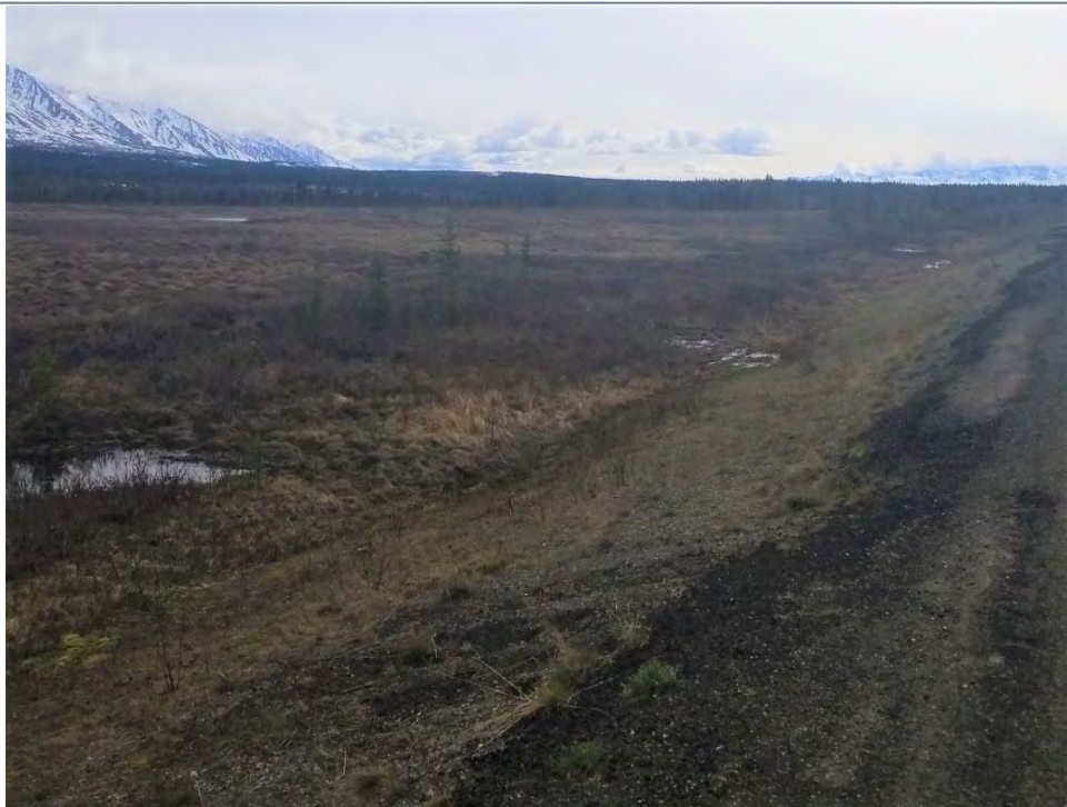
Photo 2: MP 208.2 to 209.3 Thaw ponds at toe of embankment slope. Thickened asphalt due to repeated patching.
