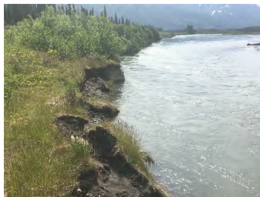
Figure 54. Erosion Just North of MP 223 Looking South (Upstream of the Nenana River)
