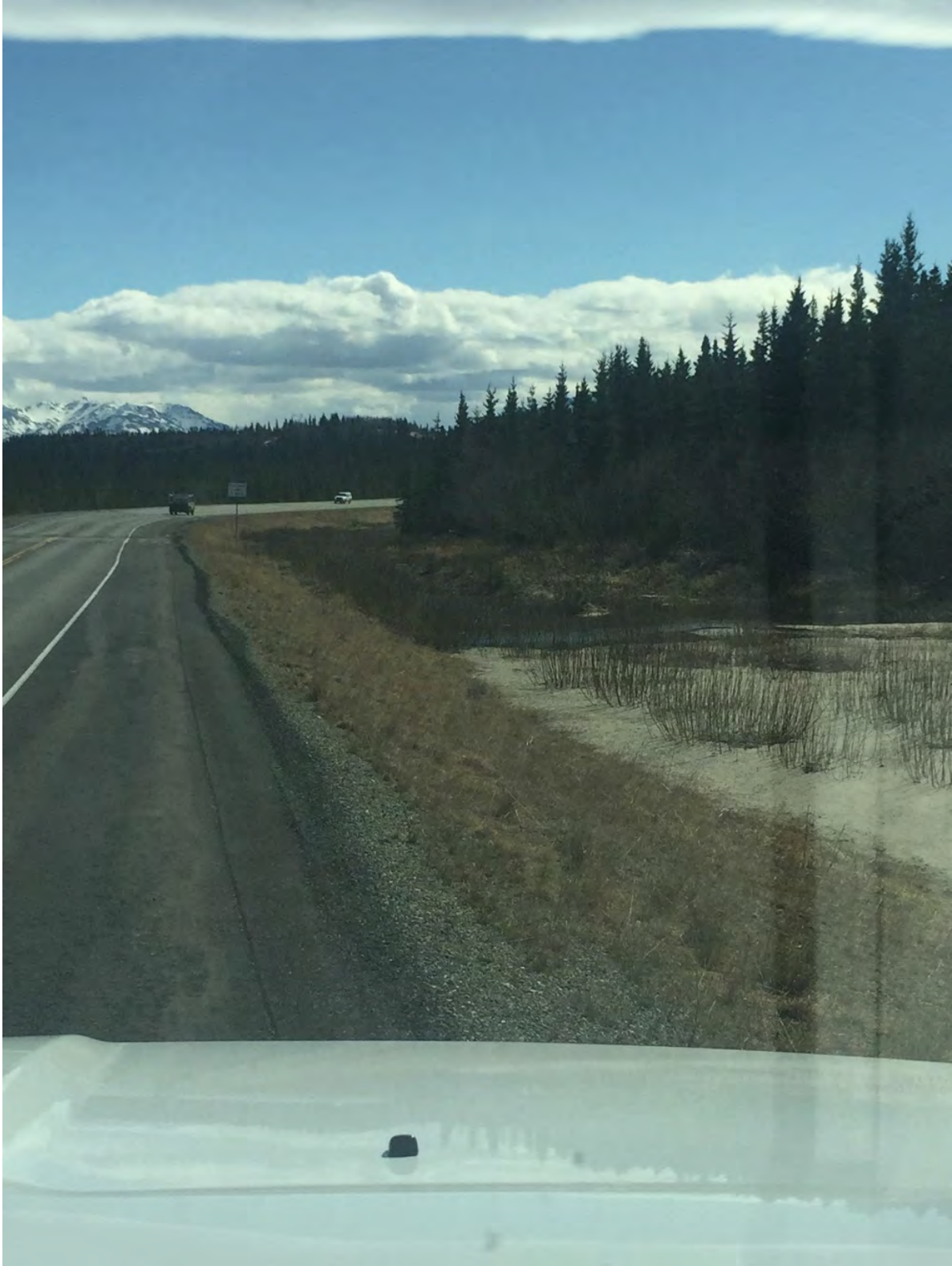
Figure 22 – Drainage issues effecting the road base near MP 258.5
