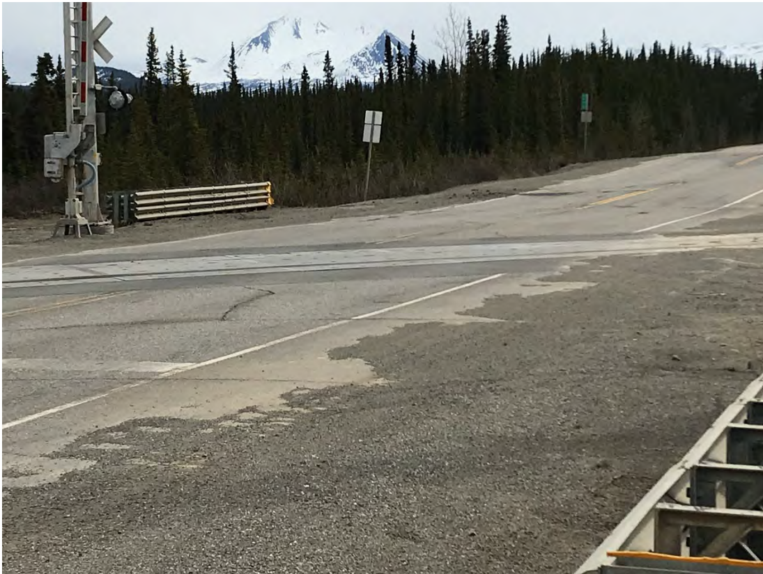
Figure 11 - Additional photo of roadway damage at railroad crossing
