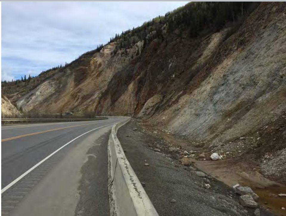
Photo 18: MP 239.2 Widened ditch with concrete traffic barrier. Some rockfall debris in ditch.
