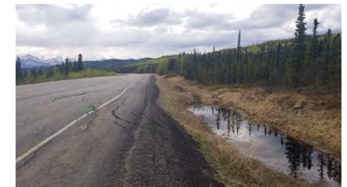
Drainage issues, roadway bumps and damage, thaw settlement (~MP 256)
