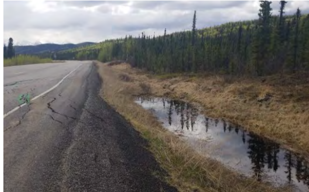
Figure 51. Ponding Observed on the Upstream Side (West Side) Near MP 256.5
