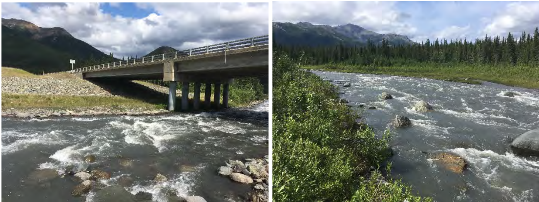
Figure 15. Riley Creek Looking Downstream, At Left Abutment, Looking Upstream from Left Abutment
