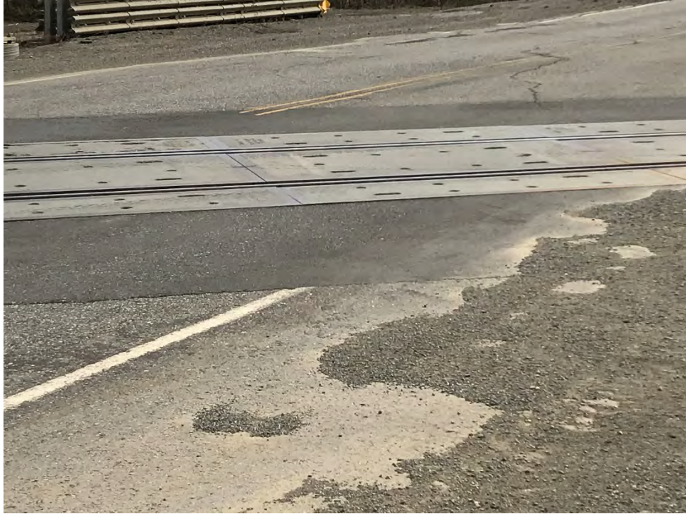
Figure 10 - Surface patches along railroad crossing
