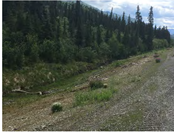
Figure 58. Roadside Ditch Low Point on the West Side Near MP 242.1
