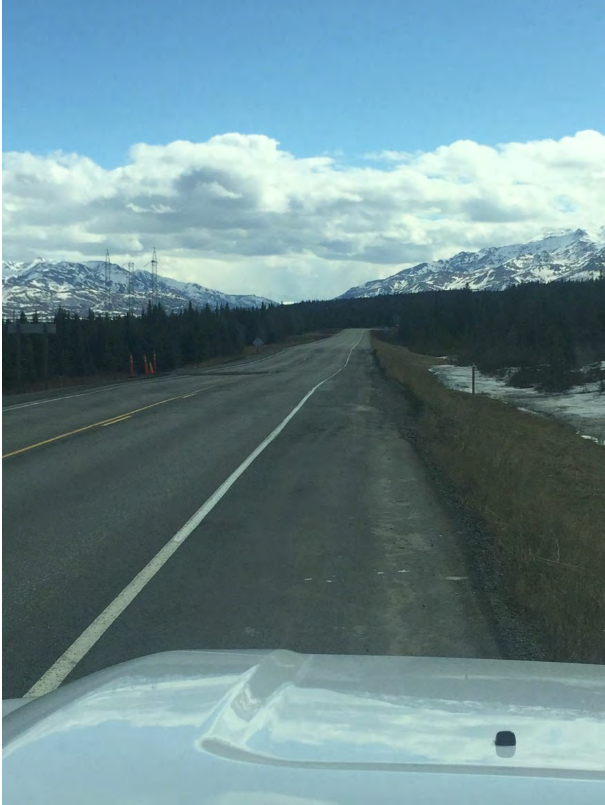
Figure 20 – Damage to road caused by drainage issues north of MP 253
