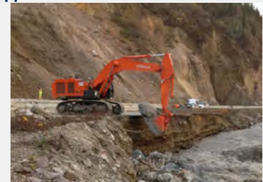
Rockfall, drainage, and sediment build up are continuous issues along the highway in Nenana Canyon (MP 239-240)
