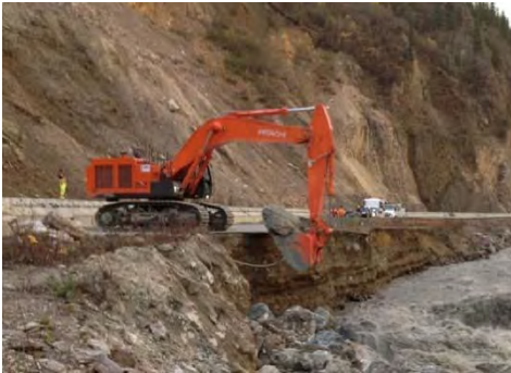
Drainage issues along the highway in Nenana Canyon (MP 239-240)
