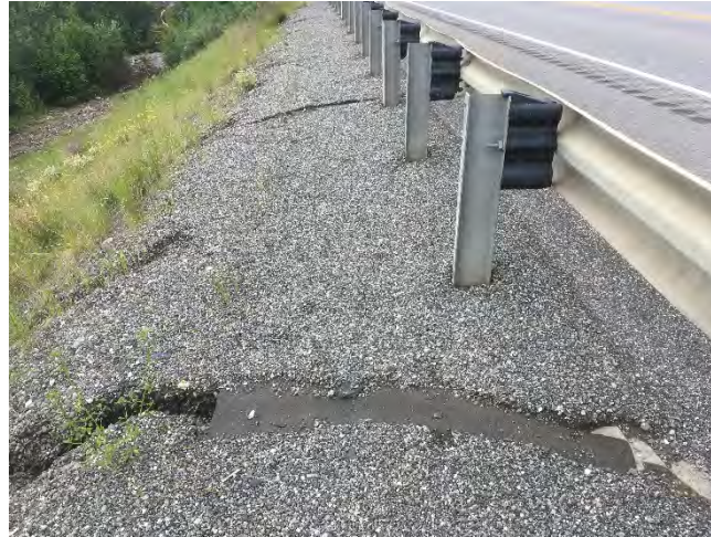
Figure 61. Shoulder Erosion Near MP 252.5 Looking South Towards the Panguingue Creek Crossing
