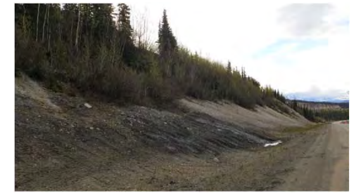
Unstable cut slopes (~MP 238)
