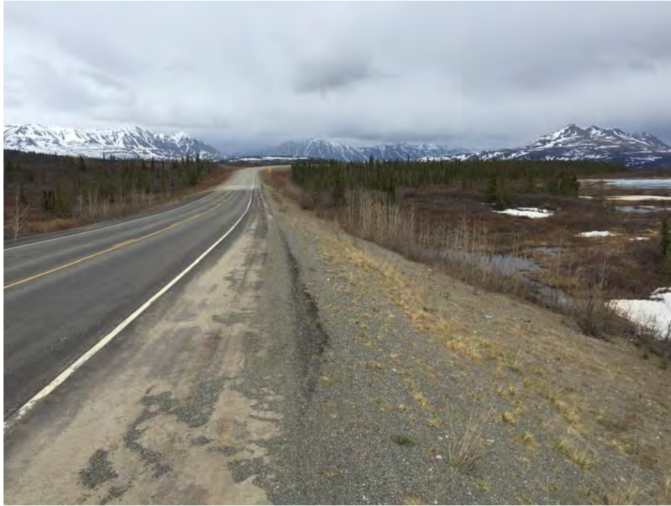
Photo 1: MP 206.2 to 206.3 Road bumps where embankment crosses a low spot between ridges. Settlement likely caused by compressible organics and thawing permafrost.
