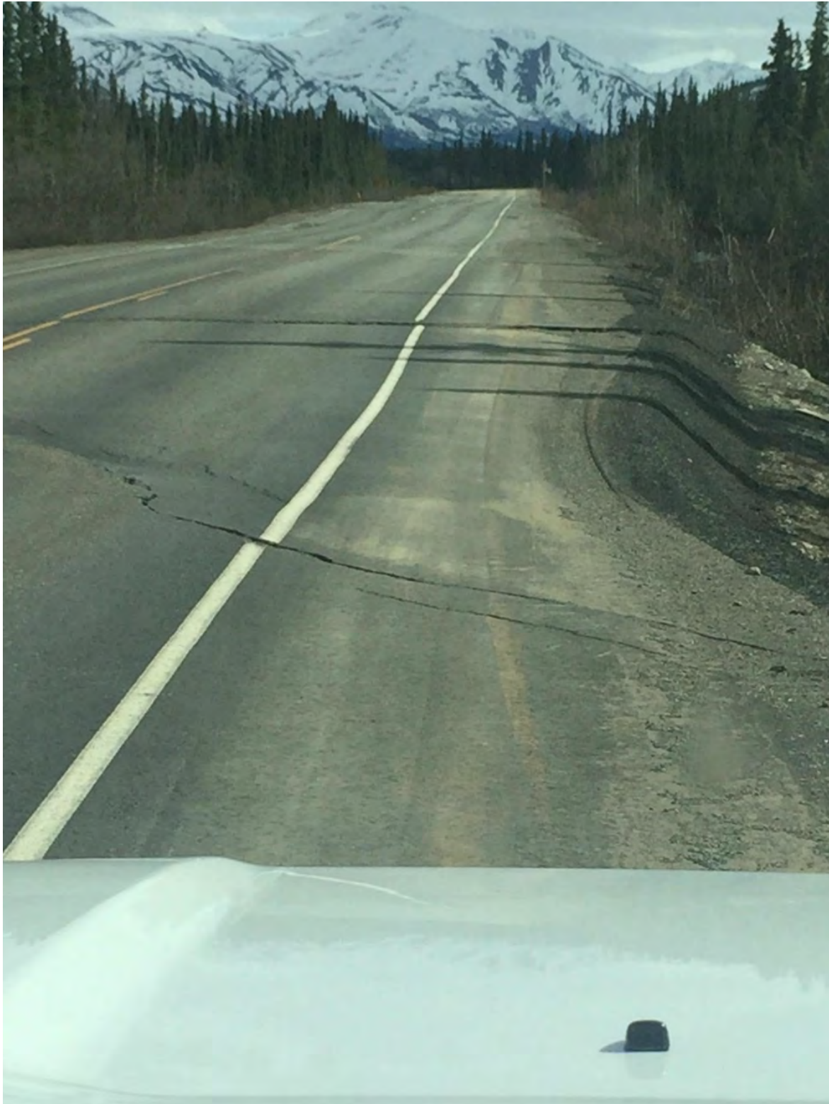
Figure 12 – Drainage issues and damaged pavement around MP 235.5
