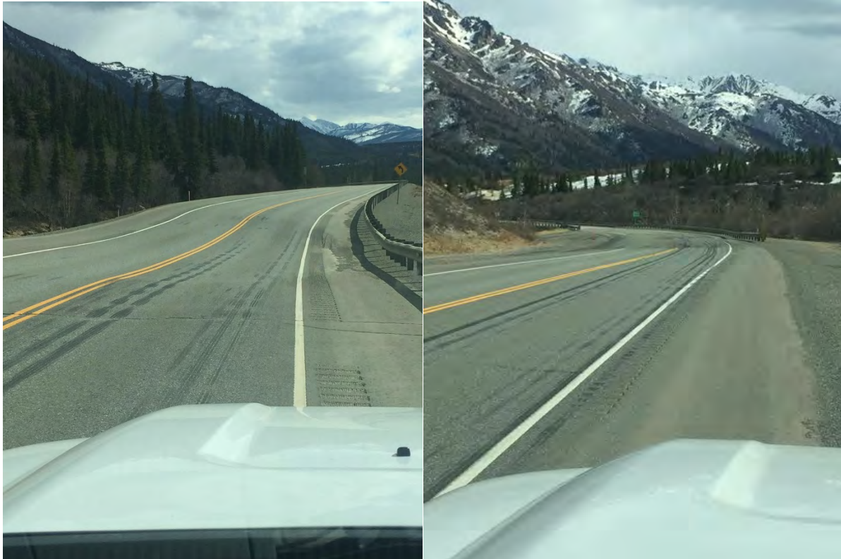
Figure 19 – Sinking roadway around MP 242 (left) and MP 243.5 (right) of the Parks Highway
