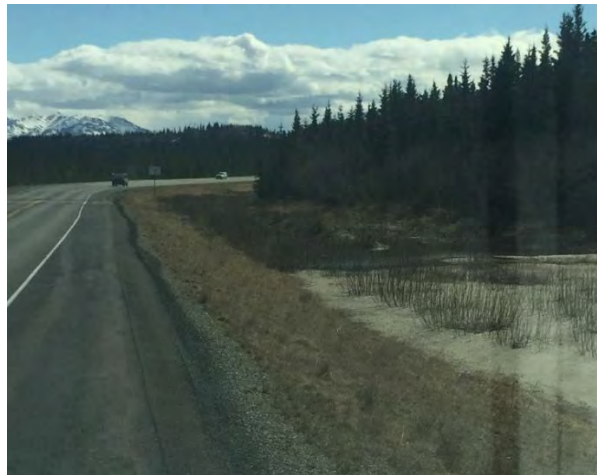
Figure 52. Ponding Observed on the Upstream Side (West Side) Near MP 258.5
