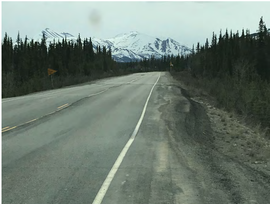
Figure 14 – Additional photo of section requiring annual maintenance due to drainage issues
