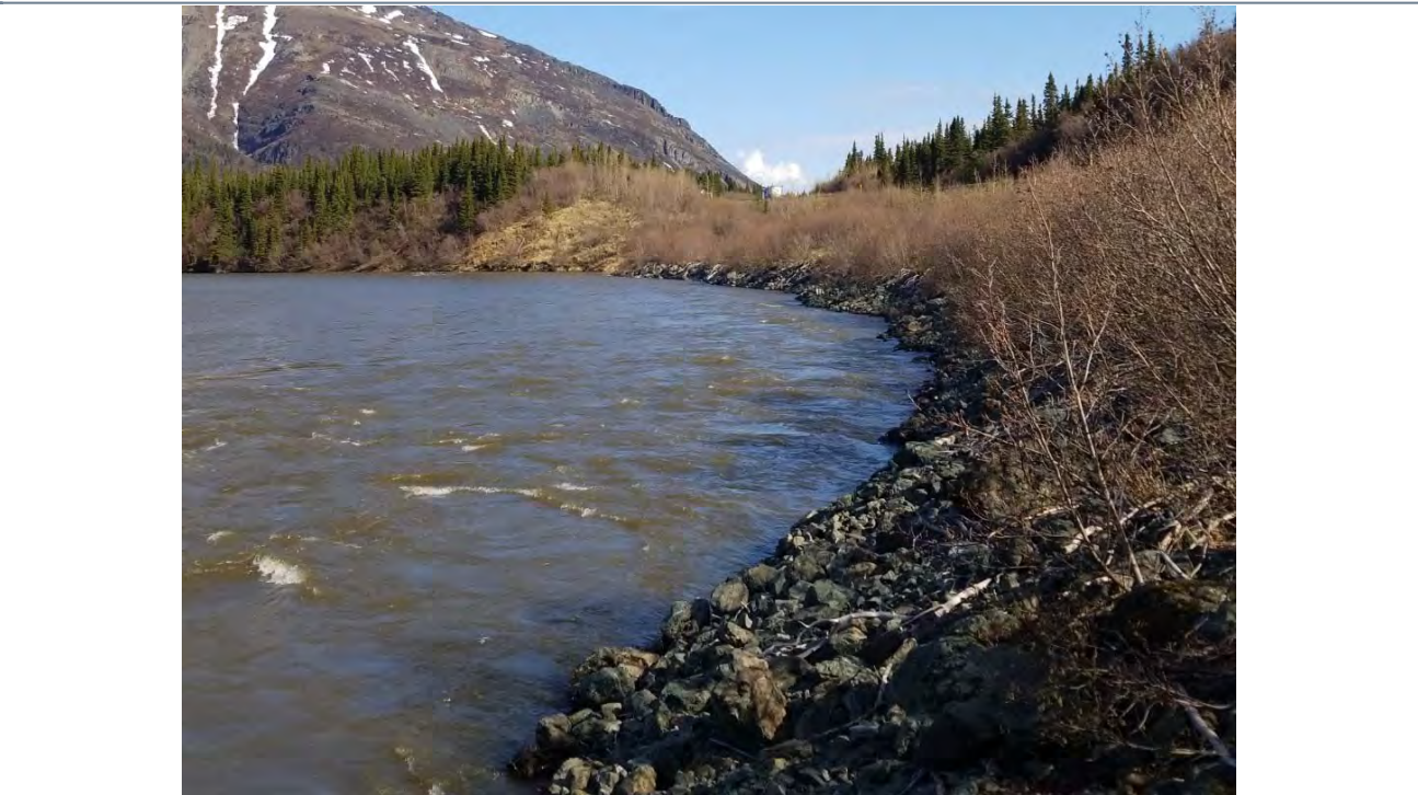
Photo 8: MP 219 Existing erosion protection along the Nenana River.
