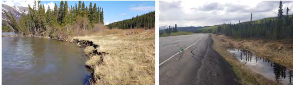
Bank erosion from Nenana River adjacent to the Highway (MP 222.8) (Left), Roadway deterioration adjacent to thaw pond, likely caused by thawing permafrost (MP 256.4) (Right)
