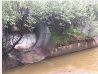
Culverts at Slate Creek (MP257.8), shown here, and Little Panguingue Creek (MP 254) are identified by ADF&G as poor for overall fish passage
