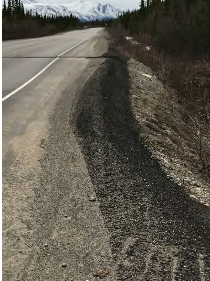
Figure 13 – Section of highway that requires annual repairs around MP 235.5
