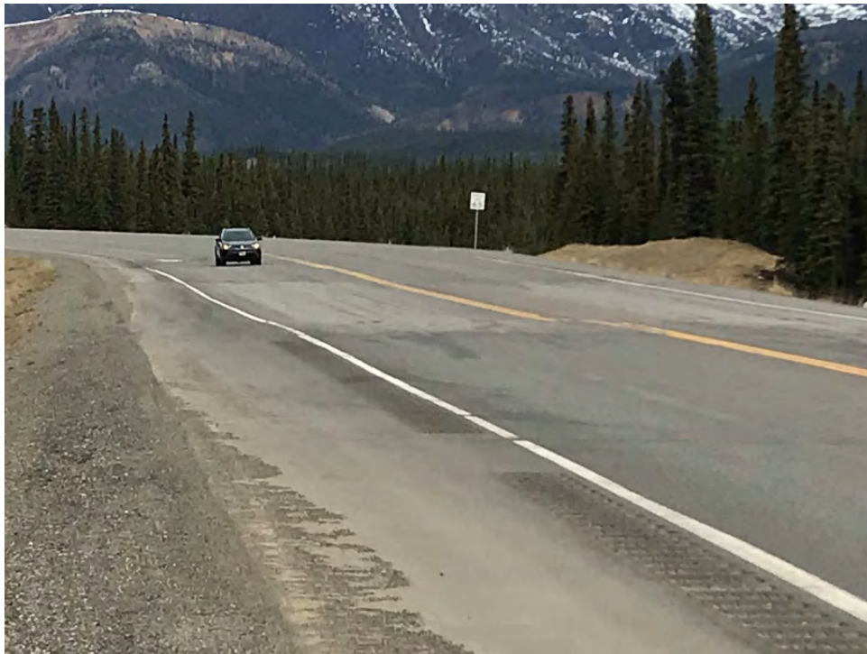
Figure 8 - Annual maintenance for pavement and roadway integrity issues near MP 232.7
