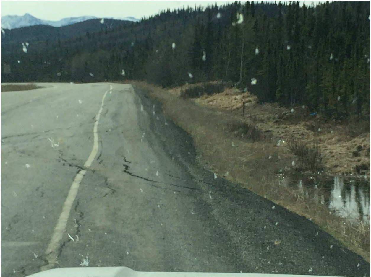
Figure 21 - Road shoulder failing due to drainage issues around MP 256.5
