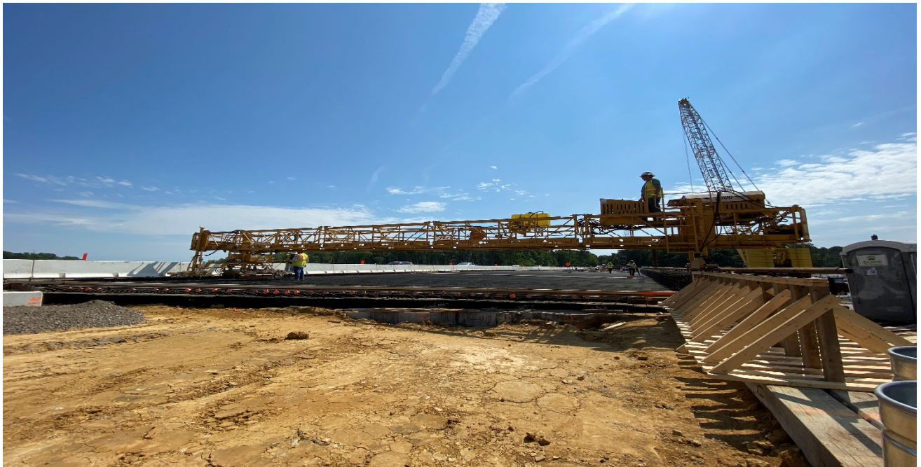
Concrete Bidwell being setup into place in preparation for scheduled concrete deck pour. (Facing East)
