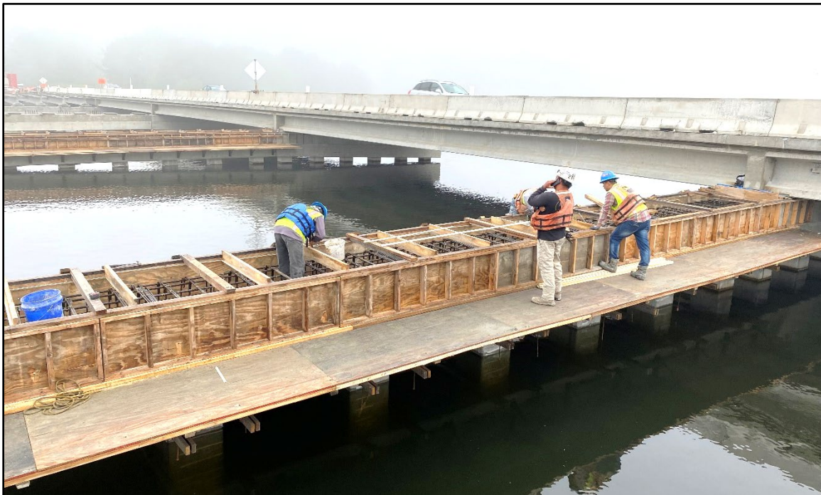
Checking Formwork and Steel Placement in Preparation for Bent Cap Concrete (Looking West)
