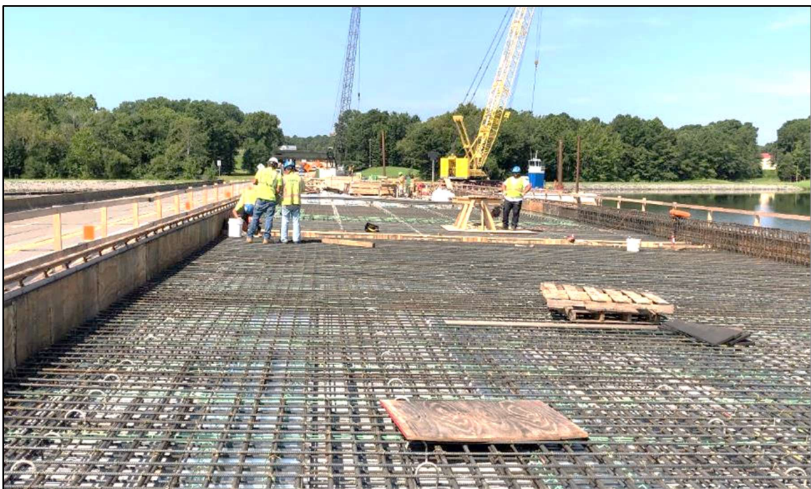
Bridge Deck Reinforcing Steel Placement in Preparation for Deck Concrete (Looking West)
