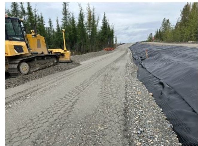
Below: Borrow Type B install on Lathrop St. between Northlake and the levee.
