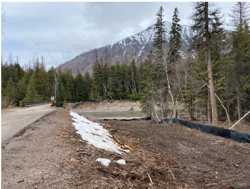
East end of the new Upper McDonald Bridge alignment looking west along
