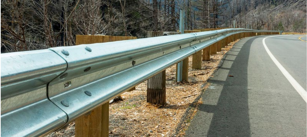
Figure 7. Example safety-only improvement (guardrail). Source: ODOT Flickr 2024.
