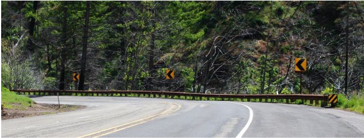
Figure 8. Example of Guardrail with Weathering Agent along OR 138 near Susan Creek Campground. Source: FHWA 2022
