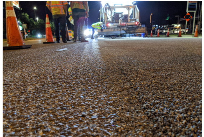
High Friction Surface Treatment is applied by a night work crew. Photo courtesy of FDOT.
