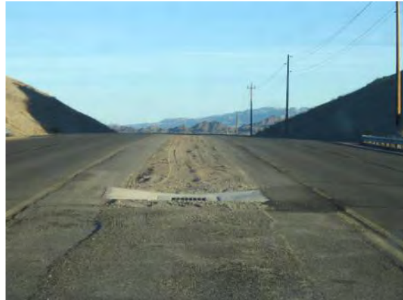
Raised traversable median drains.
