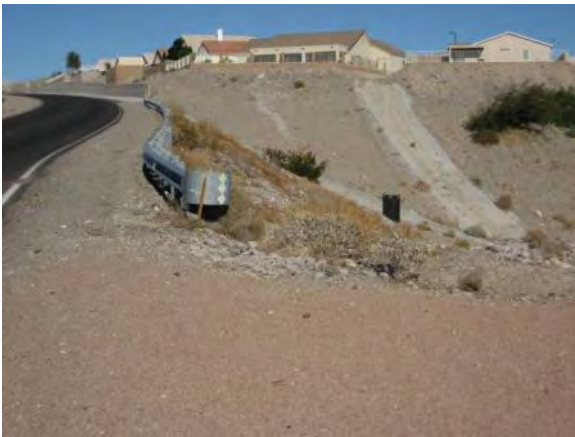
Out-of-date end terminals.
