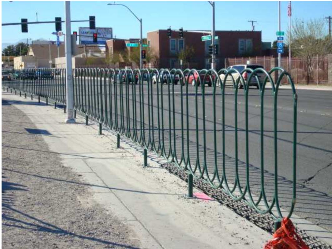
Figure 27: Pedestrian Channelization installed at Site 9/10
