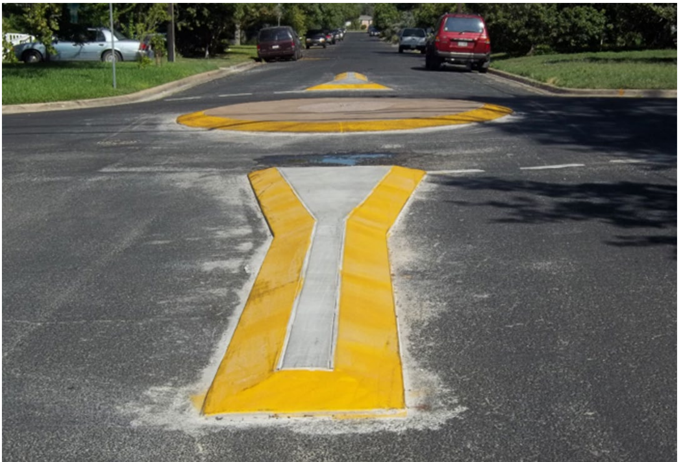
Images of several physical engineering countermeasures used are shown above: Rain Garden Bulb Out (top left), Median and Speed Cushions (top right), and Mountable Traffic Circles (bottom). Source: City of Austin
