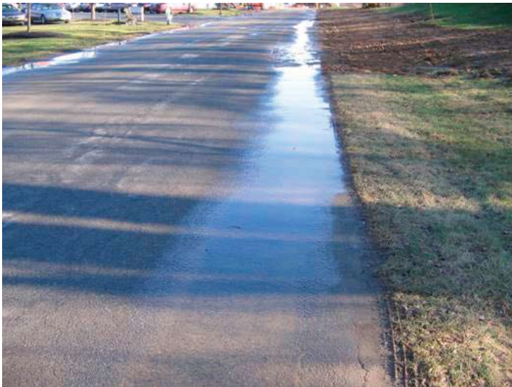
High shoulder due to vegetation growth on the shoulder prevents water from running off of the pavement, saturating the road base and causing safety problems such as ponded water (and ice in the winter).
