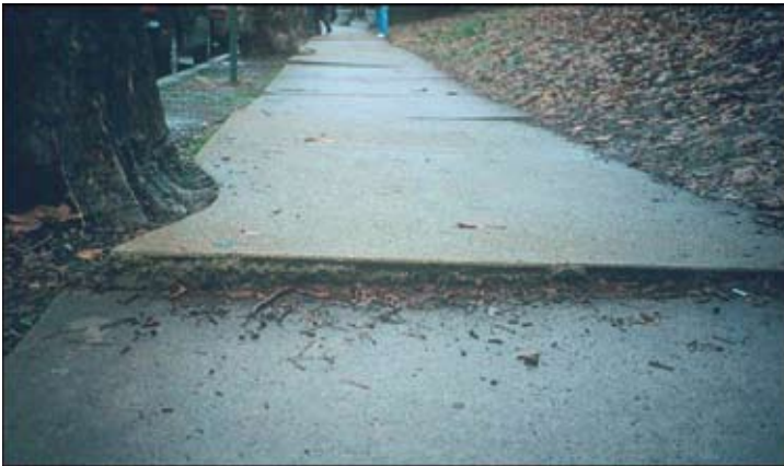
This change in level in the sidewalk due to tree roots creates a pedestrian tripping hazard and makes the sidewalk inaccessible to wheelchair users.
