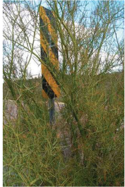
This object marker and culvert headwall are almost completely obscured by dense vegetation.
