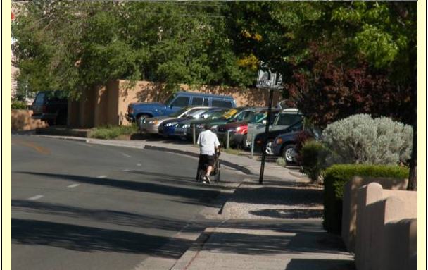
Photo shows a sidewalk along Cordova Road where the surface has deteriorated. The RSA team observed a person pushing another person in a wheelchair along this section; however, they had to push the wheelchair in the roadway due to the condition of the sidewalk surface.
