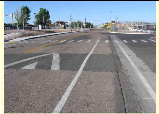
View along access road to train station. Photo shows where a speed hump extends into the bicycle lane. This presents a hazard to bicyclists.
