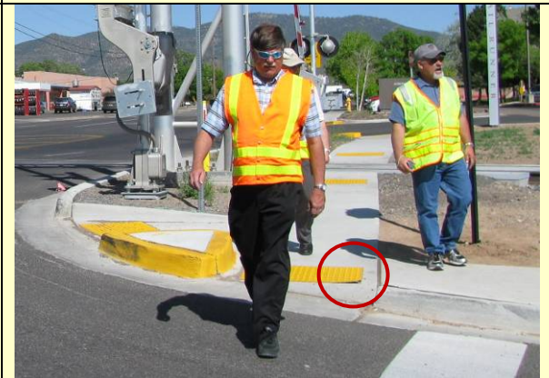
Photo shows a truncated dome that is separating from the surface of the sidewalk.
