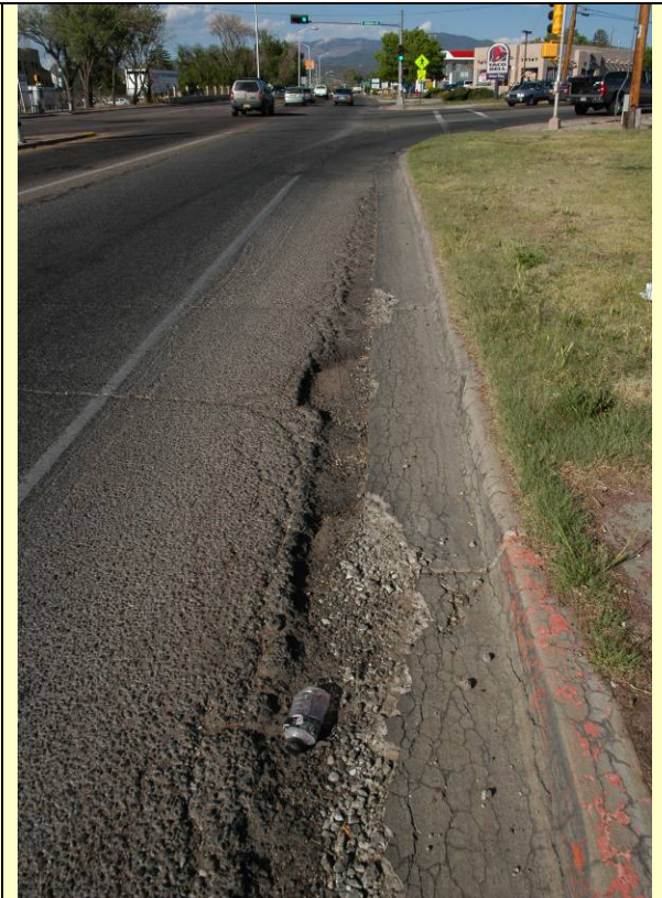
Photo shows where pavement deterioration presents a hazard to bicyclists due to the uneven surface.
