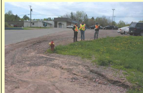
View of the southern access point at the Isle Vista Casino. Photo shows where debris from the parking lot has washed out into the ditch.
