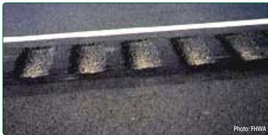
FIGURE 4. Example of Milled Rumble Strips
