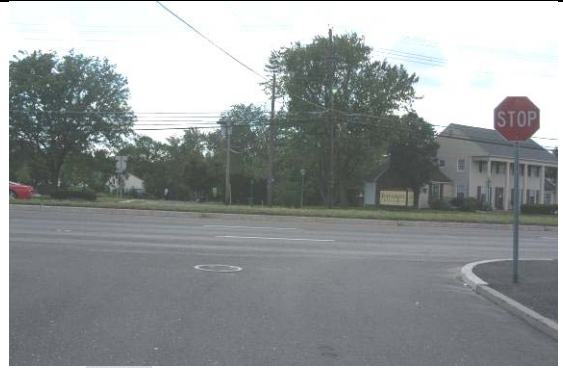
View of crossing on north side of intersection at Union Ave. Note that there is no crosswalk or curb ramp. This is an example of discontinuity and could pose a challenge to those with mobility restrictions. Furthermore, there are no indications to drivers that pedestrians may be crossing.
