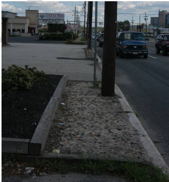
View of sidewalk along Route 70 westbound near Cornell Ave. Gaps in the sidewalk limit accessibility for pedestrians.
