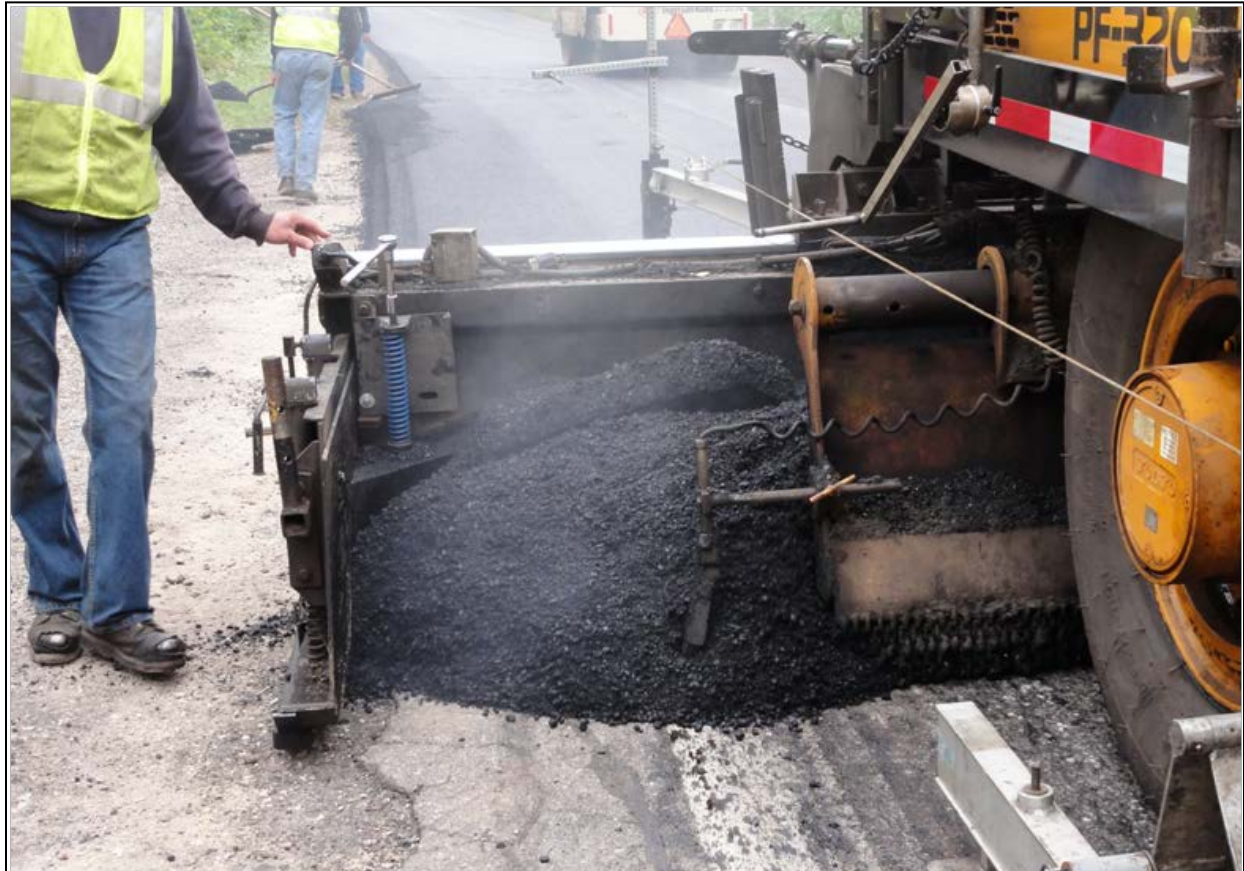
Figure 8. Paving with the Carlson prototype #2 device with the TransTech device is still attached but raised and out of the way.
