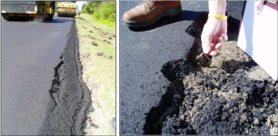
Figure 14. Isolated longitudinal edge cracking (left) and investigation revealed soil/vegetation under the pavement edge (right).
