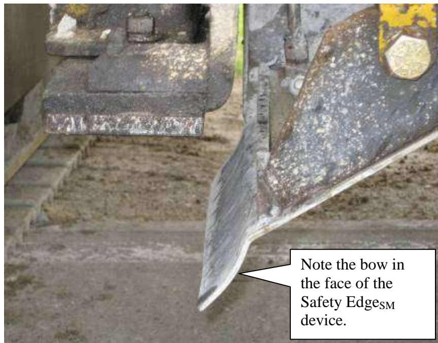
Figure 15. Viewed from the rear of paver showing the bend in the Safety Edge SM device.
