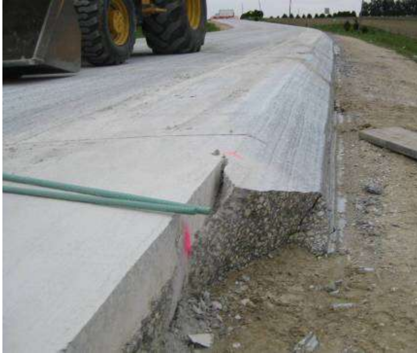
Figure 16. Saw cut edge at an intersection.
