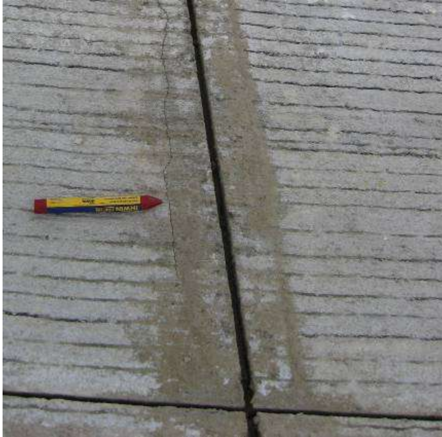
Figure 19. Random crack formed near joint.
