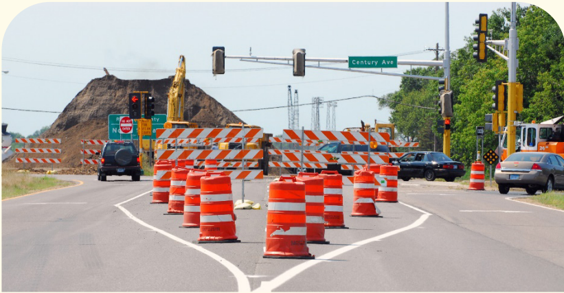
Work zones can be complex and confusing for road users. ©2007 Minnesota DOT.
