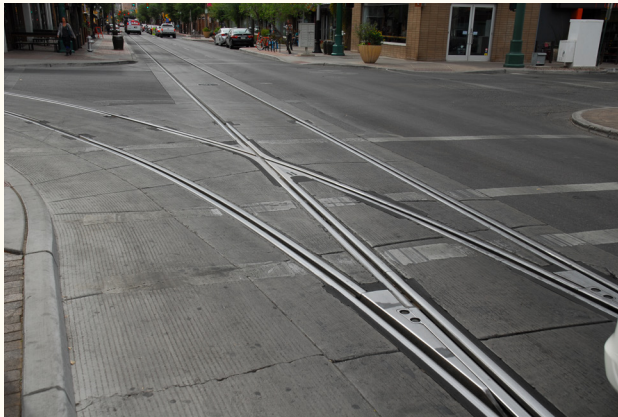
Streetcar track split can present challenges for bicycles attempting to turn left and cross over the multiple tracks (Photo credit: Dan Nabors).
