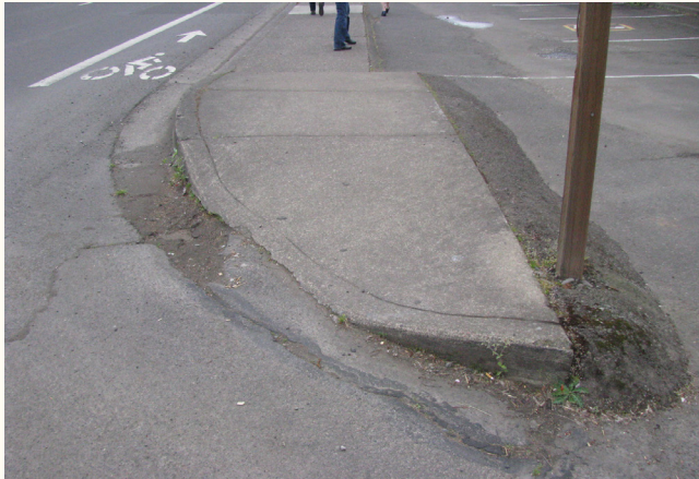
Example of ramp at an unmarked crosswalk on Main Street (Photo credit: Elissa Goughnour).
