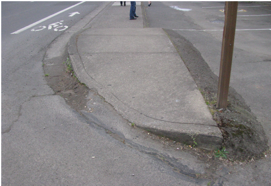
Figure 4. Example of ramp at an unmarked crosswalk on Main Street in the City of Springfield, Oregon (Photo Credit: Elissa Goughnour).
