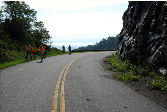
The pavement has been damaged by fallen rock and the roadway width is impacted by the encroachment of vegetation. (Credit: Dan Nabors)
