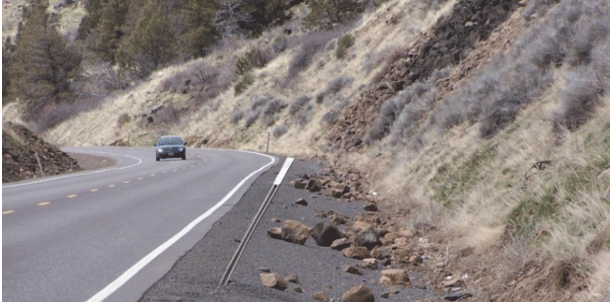
Figure 16: Rockfall in US 97 RSA Study Area.
