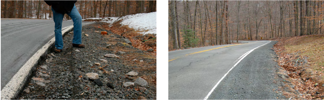
Figure 23: Shoulder with edge drop-off before (L) and after (R) RSA was conducted The edge drop-off was immediately corrected following the RSA workshop
