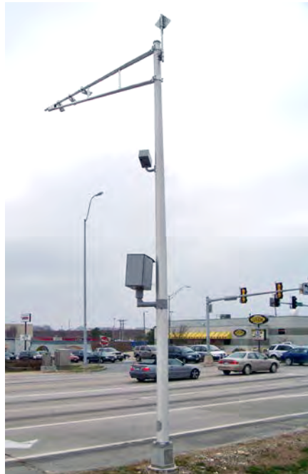
Exhibit 2-8. Enforcement cameras, as shown in the photo above, are used at signalized intersections to identify red light runners.
