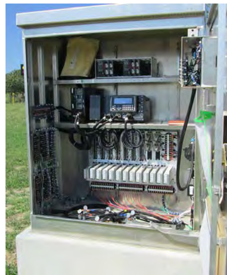
Exhibit 1-3. Inside a signal controller cabinet. Photo Credit: Missouri DOT
