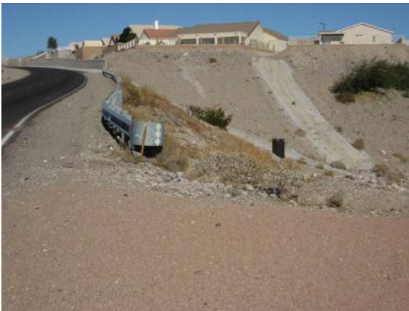
Out-of-date end terminals.
