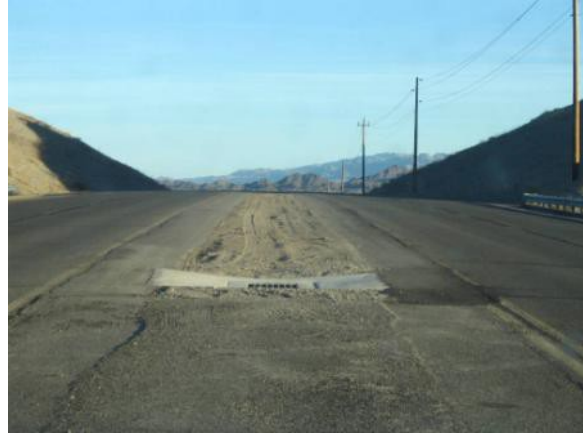
Raised traversable median drains.
