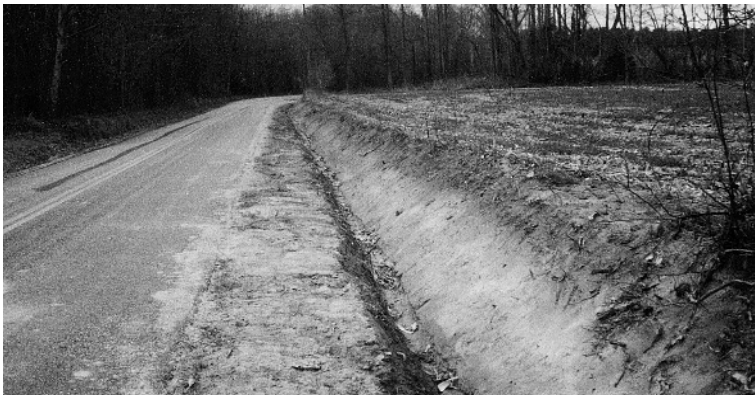
This regraded earth shoulder and ditch has a steep backslope which makes it non-traversable; if right-of-way is available the backslope should be made less steep.
