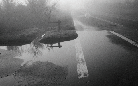
In this photo, water is ponding because the outflow ditch has silted up. Ponded water can cause drivers to leave their lane, reduce braking ability or contribute to pavement deterioration.
