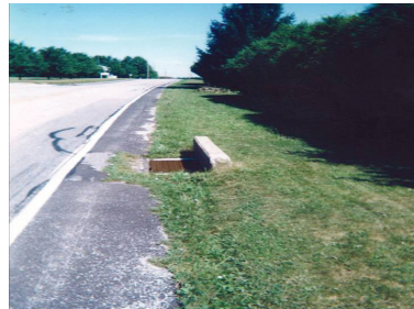
The headwall is sticking up almost a foot in a relatively flat recoverable area. It can snag a vehicle and bring it to an abrupt stop or cause it to overturn.
