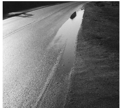
Water ponding at the edge of roadway.
