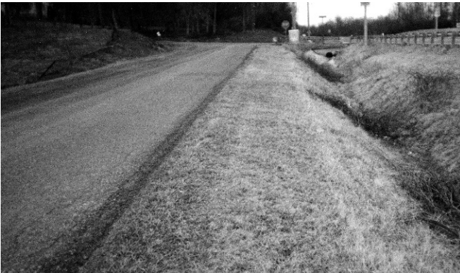
Side slope erosion can cause rollovers.
