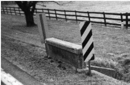
This headwall is a roadside obstacle and should be replaced as soon as possible.
