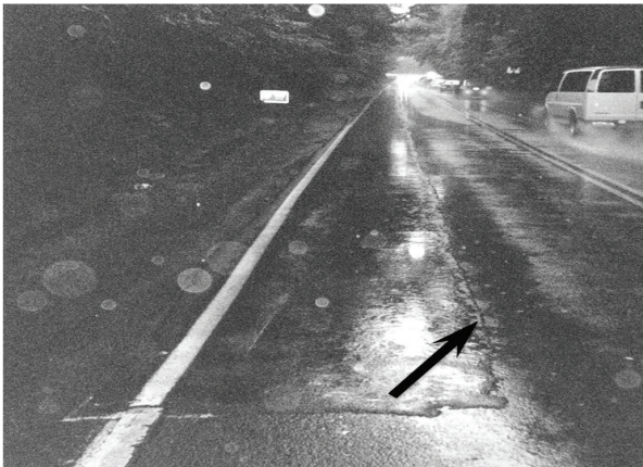
The edge of this partial pavement overlay is causing water to be retained on the travel way surface.
