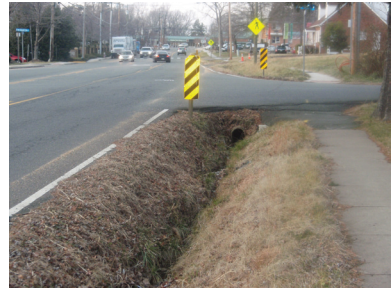
A non-traversable drainage ditch such as this is a safety hazard.
