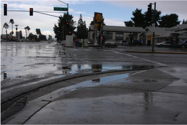
Water standing in the roadway.
