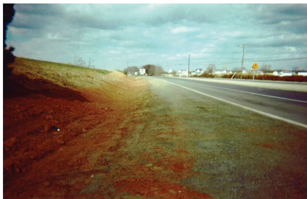
This ditch was reshaped to provide a safe recovery area for errant vehicles.
