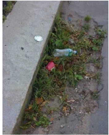
A clogged drain can easily be detected during a field survey.
