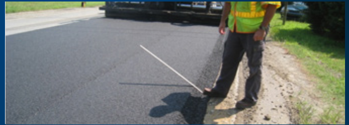
Figure 6. Paving a Delaware roadway with SafetyEdge SM . After paving, a graded shoulder will become flush with top of the pavement, covering the sloped edge. Source: FHWA.
