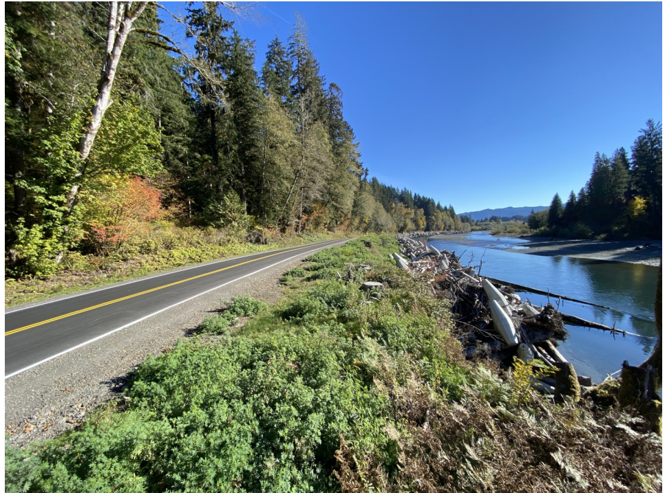
New asphalt pavement and striping (Left), Willow plantings and native species seeded area (center), Engineered Log Jams with Dolosse (Right)
