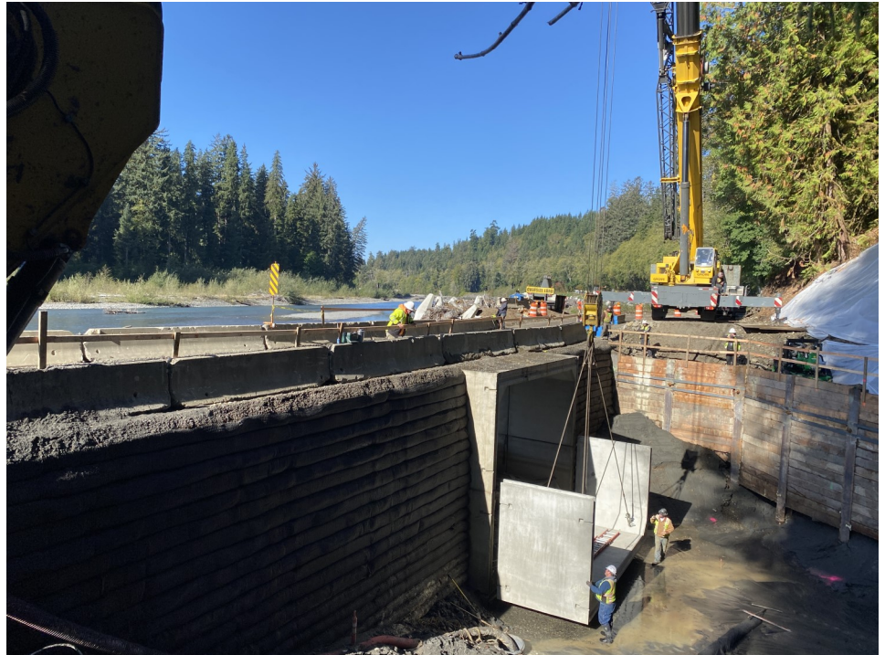
Installation of the inlet half of the MP 4 culvert. The culvert is 18ft tall. The section of culvert being placed in this photo weighs 45,000 lbs.
