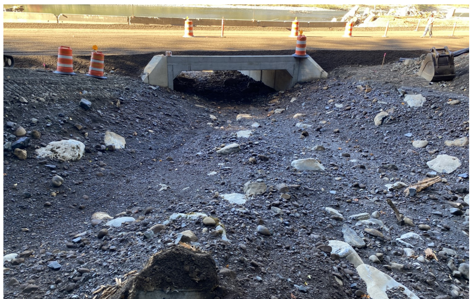
The MP 4 box culvert is backfilled and the stream channel is reconstructed through the culvert. Paving is scheduled for this week.
