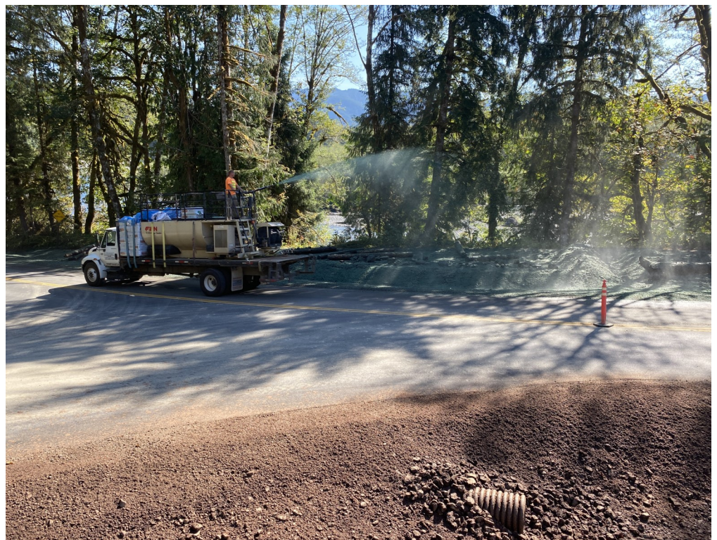
Hydroseeding at Tower Creek. Applying green mulch second application. (First application of brown-colored soil, seed, fertilizer mix in foreground)
