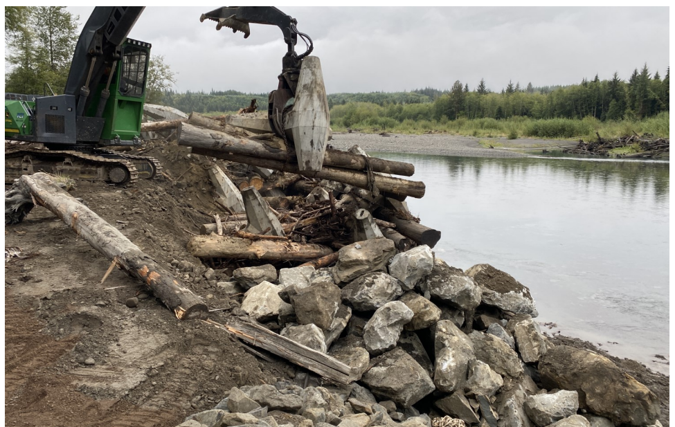
Reassembly of the ELJ #23, which was partially disassembled to facilitate installation of the outlet sections of the MP 4 box culvert
