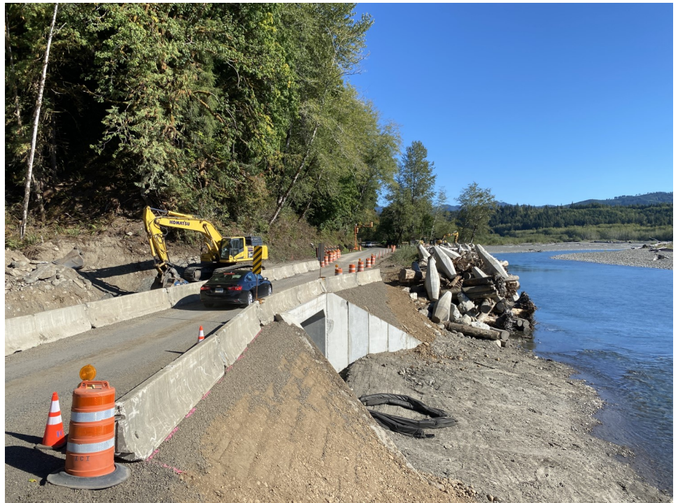
Temporary bypass lane shifted to the south side of the road, over the newly installed culvert
