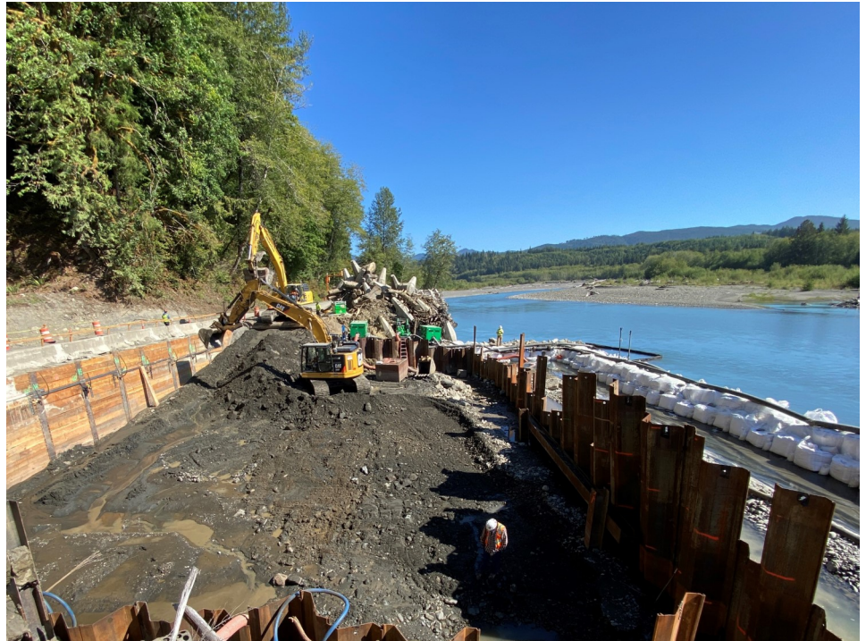
Temporary Shoring Wall (Left) and Hoh River work isolation and flow diversion system (Right). Excavation to box culvert foundation elevation
