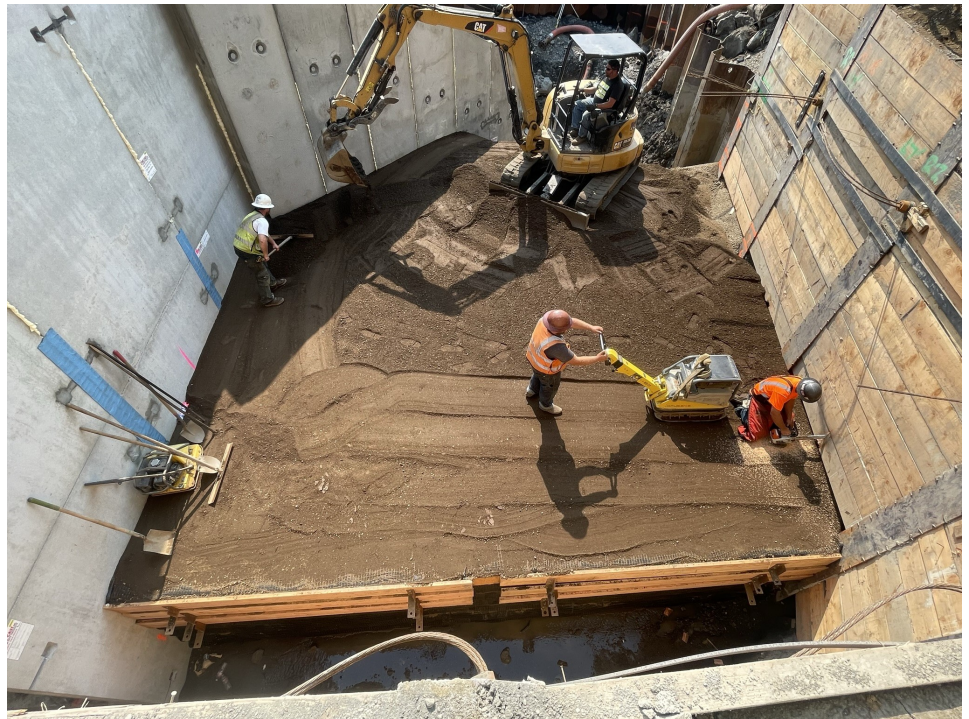
Backfill of box culvert: placing borrow material, compacting, removing timber lagging shoring wall as backfill progresses upward
