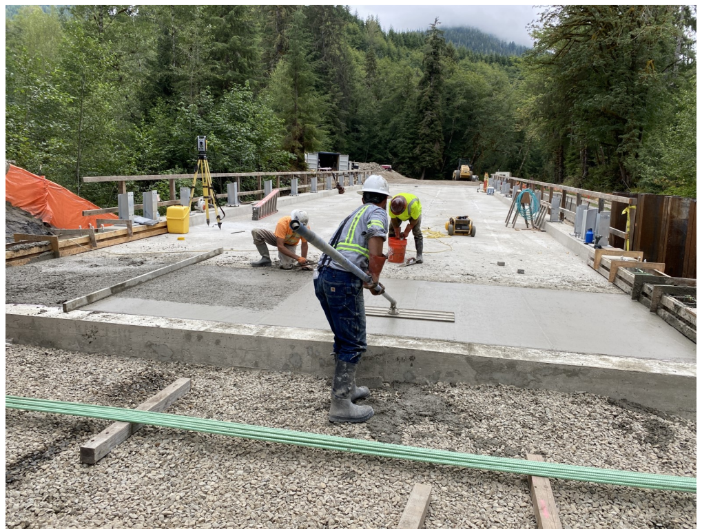
Placing and finishing the concrete for the west Tower Creek approach slab
