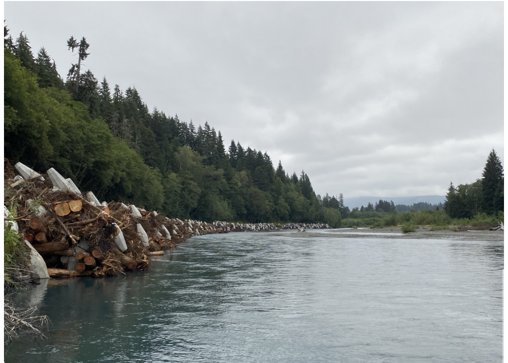
A view of some of the completed Engineered Log Jams at MP 4
