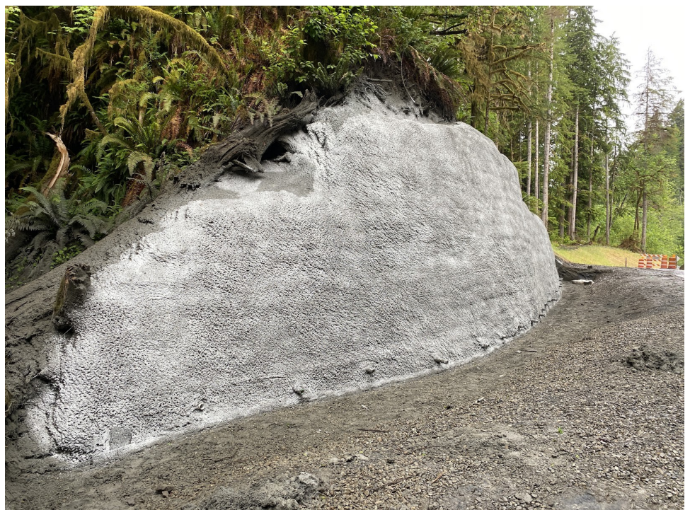
Final Shotcrete face of wall to be covered with a rockery wall
