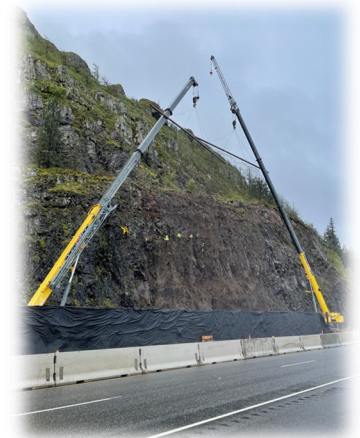
Below: Scaling at Stepped Cut
